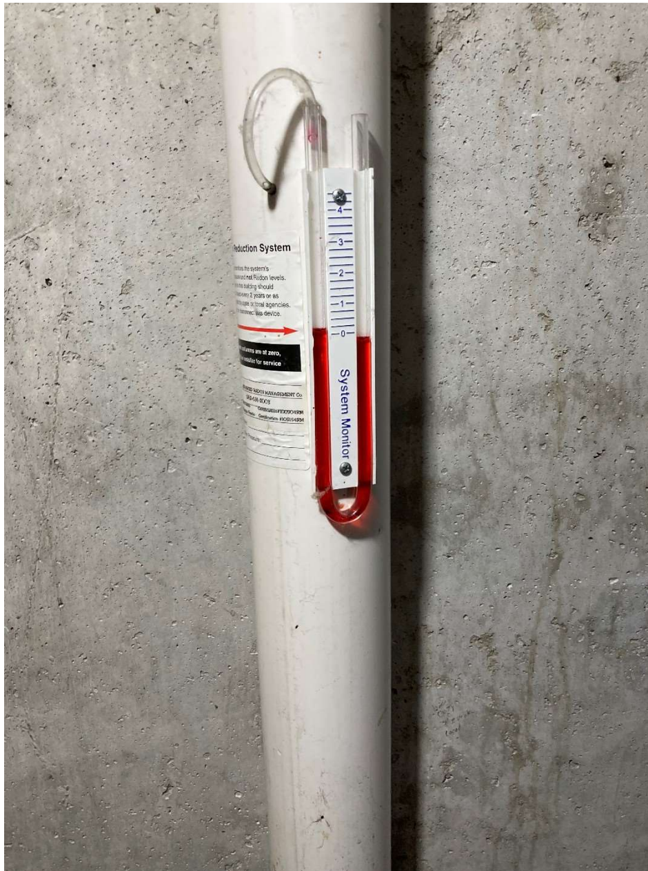
U-Tube Liquid Manometer located in building basement
