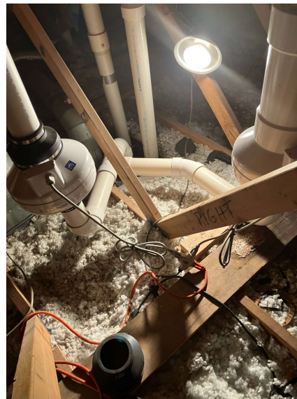
Description: Fans and power cords
