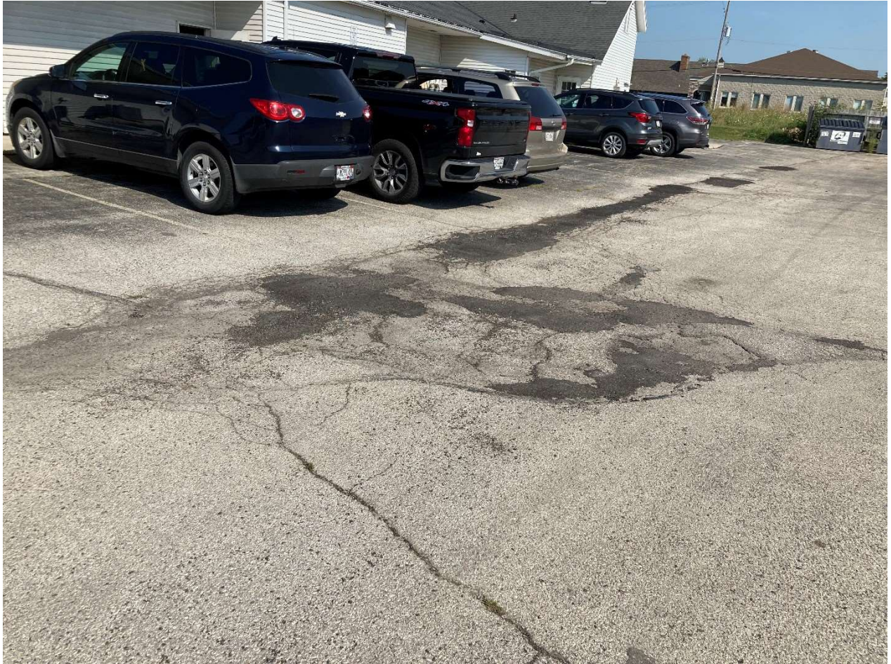
Rear (east) pavement cap – Patch work
