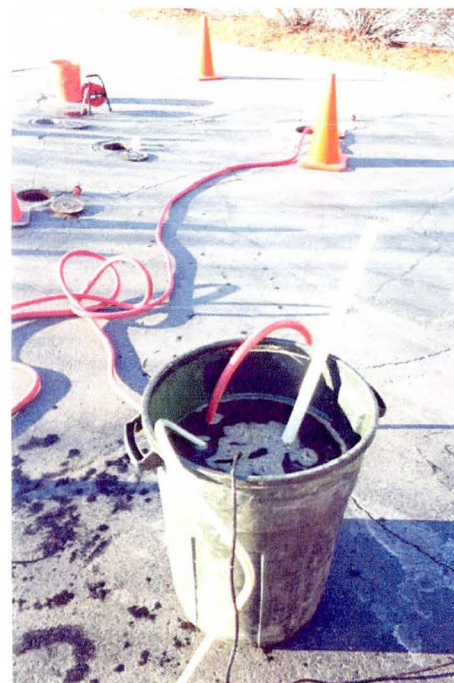
Carbon amendment solution is pumped to an injection well to enhance the biodegradation of chlorinated hydrocarbons
