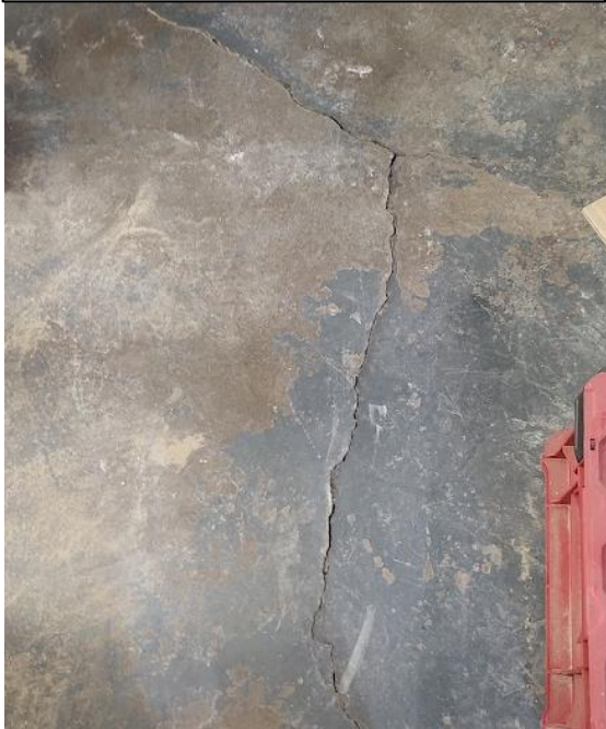
Crack in purple rectangle area.
