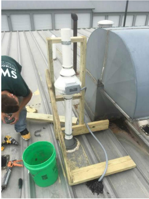
Photo #9 Photograph SDSS system installation on top of the roof (Photograph taken by SWAT).
