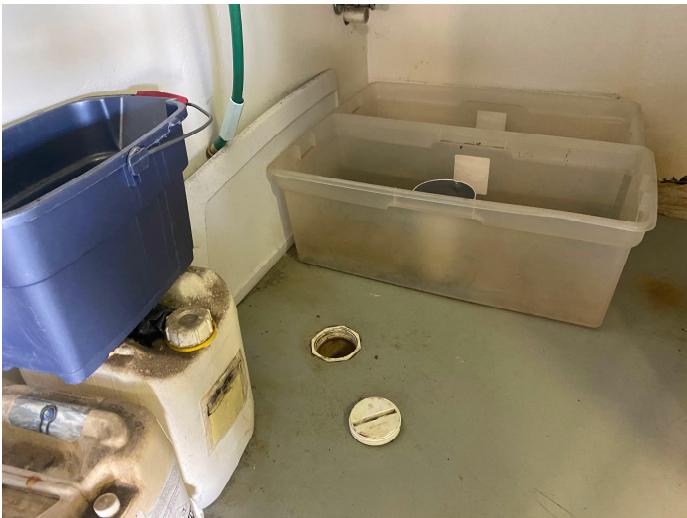
Photo #3 Approximate 4-inch diameter sanitary cleanout in the boiler room in the north part of Smoke-Out Cleaners.
