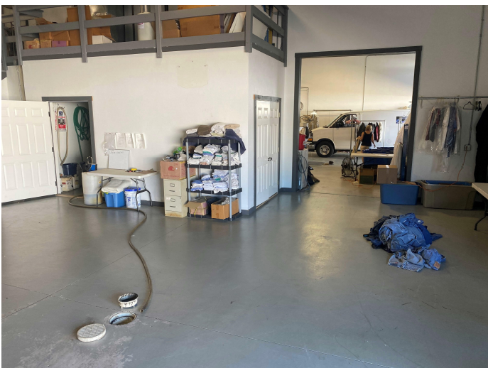
Photo #5 View of north floor drain looking south-southeast with south floor drain (through center door) and enclosed boiler room with the sanitary cleanout in upper left.
