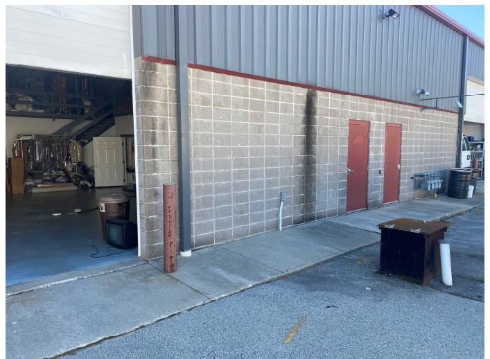
Photo #6 View from outside the north garage door looking southeast showing the north floor drain inside and the holding tank access box outside.
