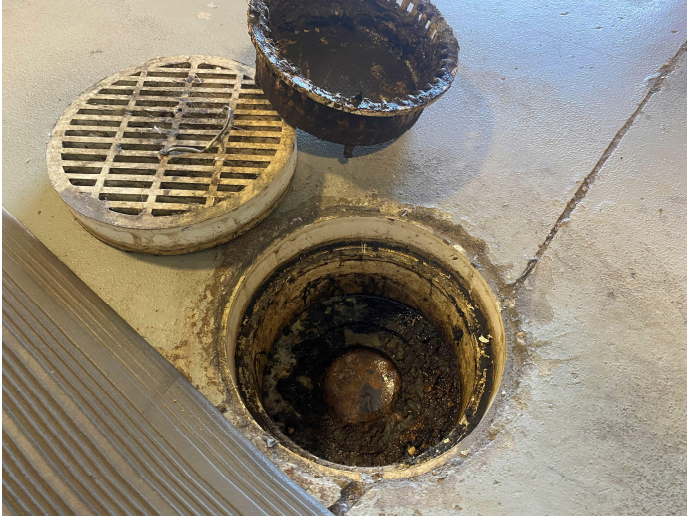
Photo #1 South floor drain plugged with sediment.
