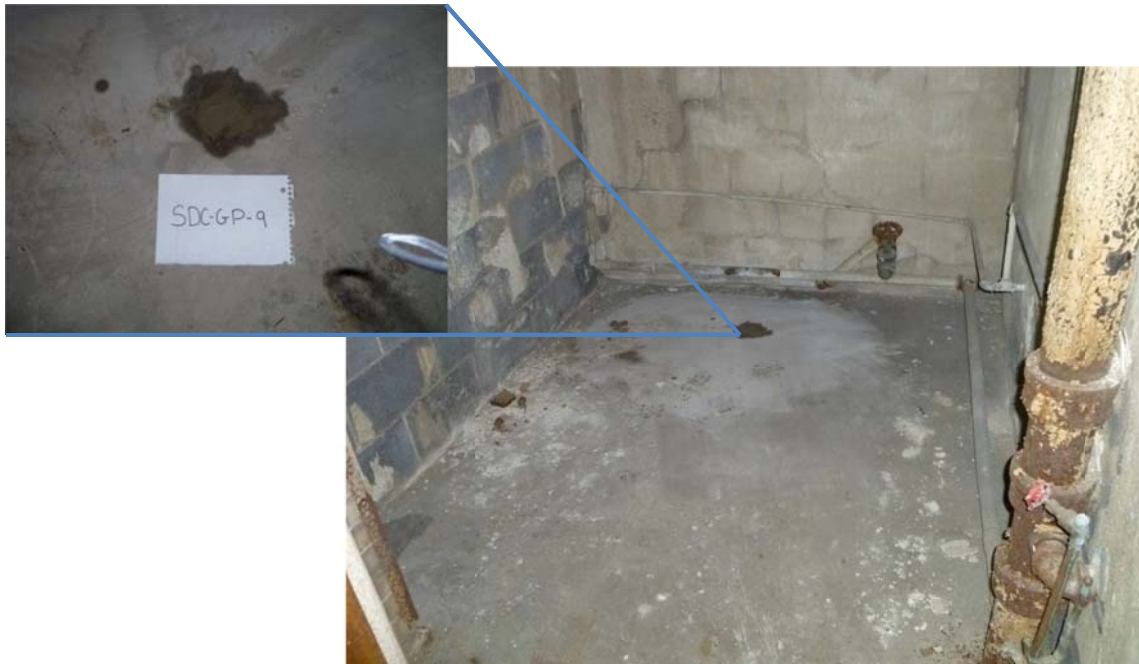
Photograph No.: 16 Photographer: Naren Babu Orientation: North TDD Number: TO-05-11-03-0007 Contract: EP-S5-10-10, OTIE Date: April 7, 2011 Site Name & Location: Sandies Dry Cleaning Site, Little Chute, Outagamie County, Wisconsin. Subject: View of the location of sub-slab soil boring SDC-GP-9 just west of the dry cleaning machine inside the site building
