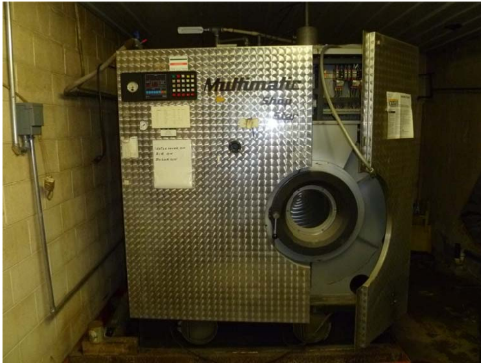
Photograph No.: 1 Photographer: Naren Babu Orientation: West TDD Number: TO-05-11-03-0007 Contract: EP-S5-10-10, OTIE Date: April 7, 2011 Site Name & Location: Sandies Dry Cleaning Site, Little Chute, Outagamie County, Wisconsin. Subject: View of the drycleaning machine located inside the wash room of Sandies Dry Cleaner site building
