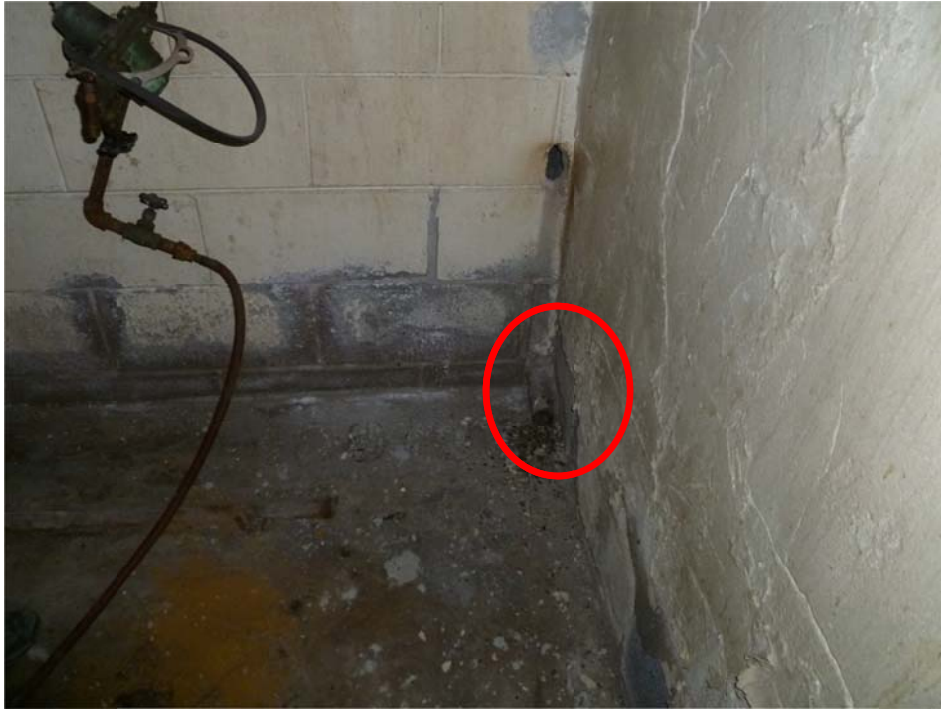
Photograph No.: 3 Photographer: Naren Babu Orientation: West TDD Number: TO-05-11-03-0007 Contract: EP-S5-10-10, OTIE Date: April 7, 2011 Site Name & Location: Sandies Dry Cleaning Site, Little Chute, Outagamie County, Wisconsin. Subject: View of the pipe in the wash room that extends to the backyard
