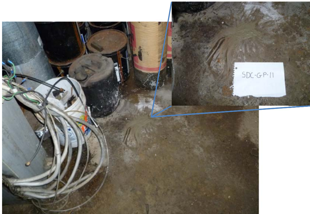
Photograph No.: 18 Photographer: Naren Babu Orientation: Looking down TDD Number: TO-05-11-03-0007 Contract: EP-S5-10-10, OTIE Date: April 7, 2011 Site Name & Location: Sandies Dry Cleaning Site, Little Chute, Outagamie County, Wisconsin. Subject: View of the location of sub-slab soil boring SDC-GP-11 in the boiler room inside the site building
