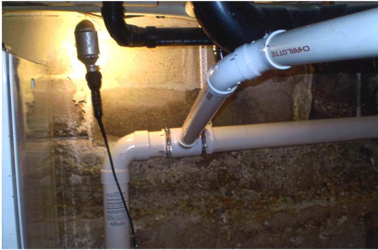
Photo 7: Looking west at drop pipe to Original Pickup Point. Pipe extends east along ceiling to Pickup Point A
