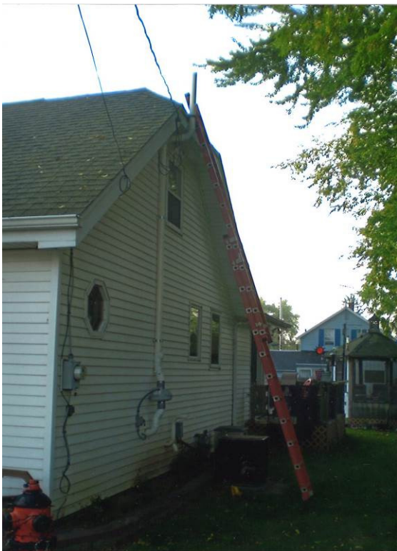
Photo 10: Looking southeast at west side of house with fan and exhaust pipe
