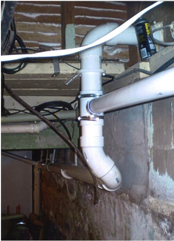
Photo 9: Looking south at piping along ceiling with drop pipe to Original Pickup Point in background. Pipe exits west side of basement to connect to exterior fan
