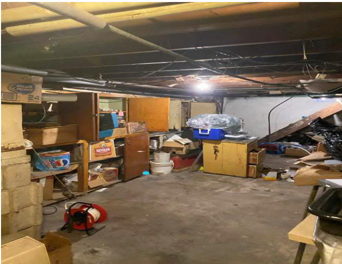
Photo #3 View of the Weenies basement area where P-2 and P-3 are located facing southwest.
