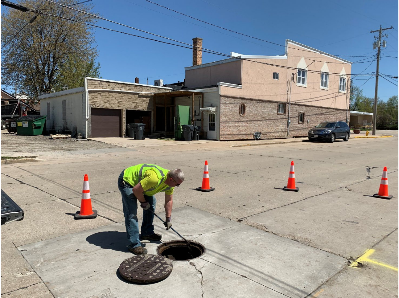
Photo 2: Accessing manhole “NHM0735/MH5” along West Lincoln Avenue with the assistance of Village of Little Chute staff.
