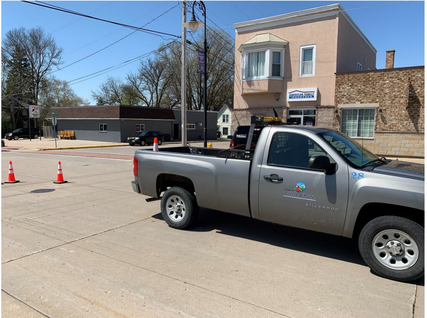
Photo 3: Accessing manhole "NMH0645/MH4" along Grand Avenue with the assistance of Village of Little Chute staff.
