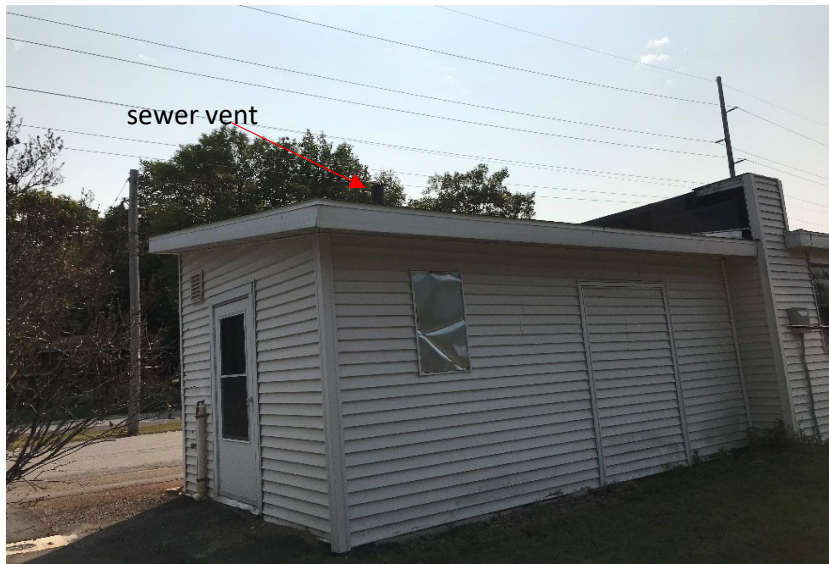
sewer vent stack on roof, northeast corner of building
