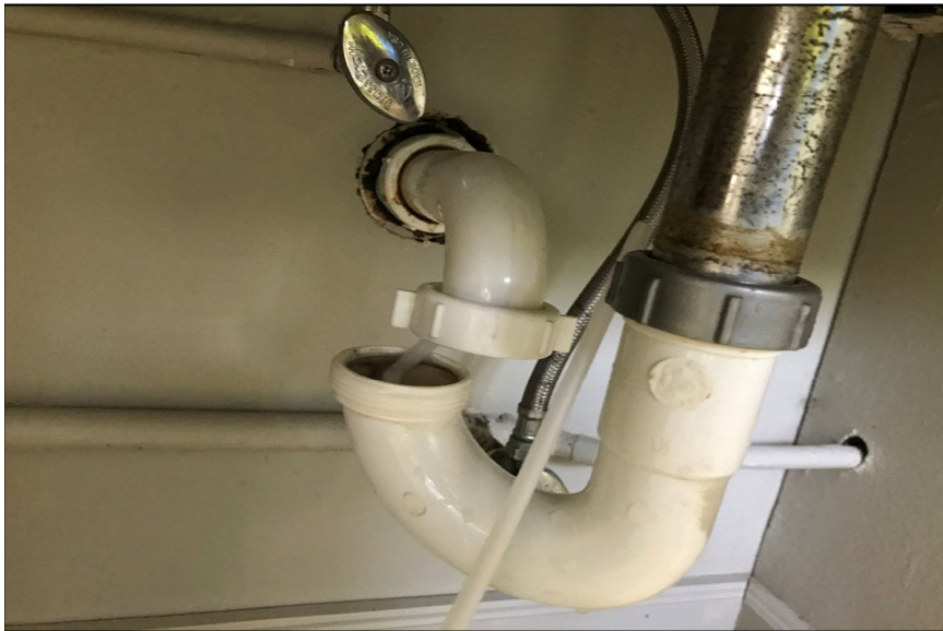
Trap disconnected to fish tubing, reconnected for sampling
