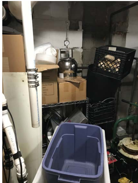
IA-4 in the Basement
