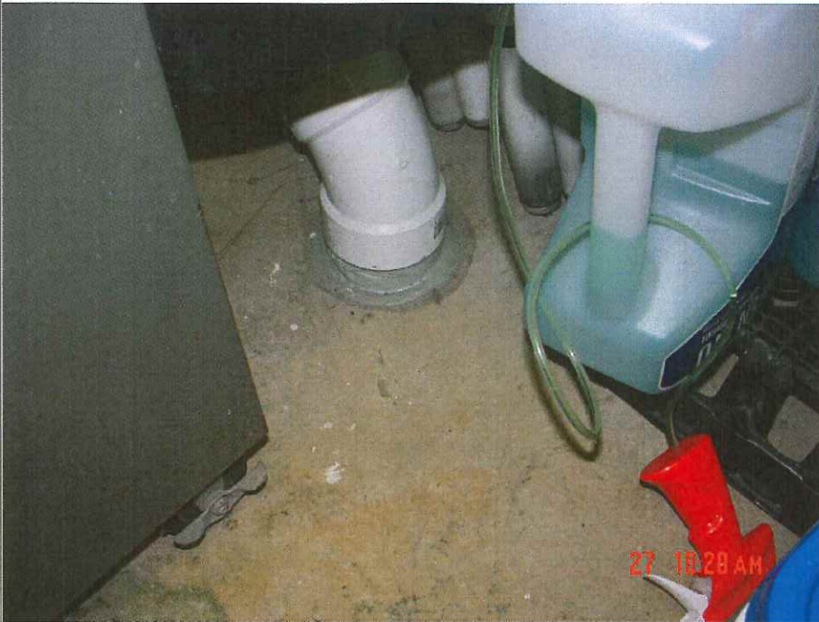
Title: Holiday Village Coin Laundry/0230553765/07272016/Piping sealed suction pint
