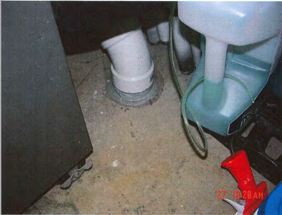
Title: Holiday Village Coin Laundry/0230553765/07272016/Piping sealed suction pint
