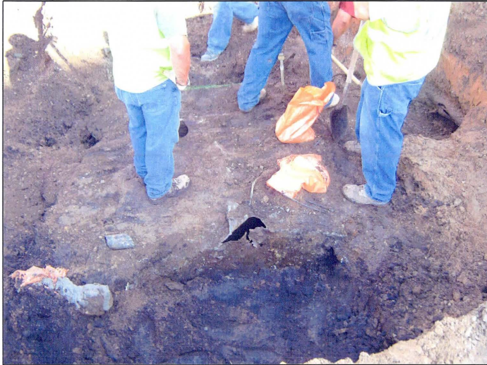
Photo 1 – Discovery of UST, Soil Staining in Foreground.
