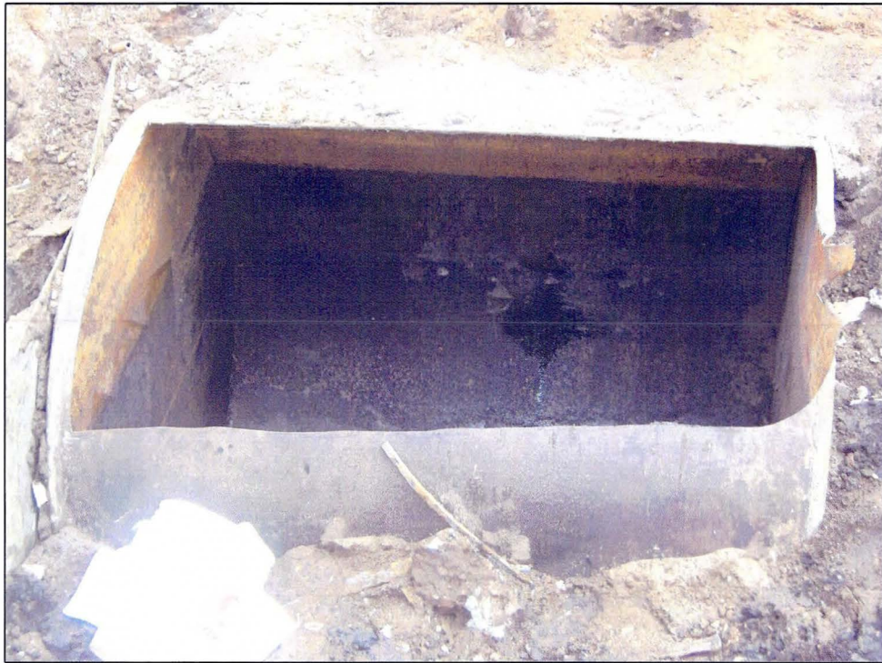
Photo 5 – Cleaned UST, Hole Observed On Back (North) Wall of UST.
