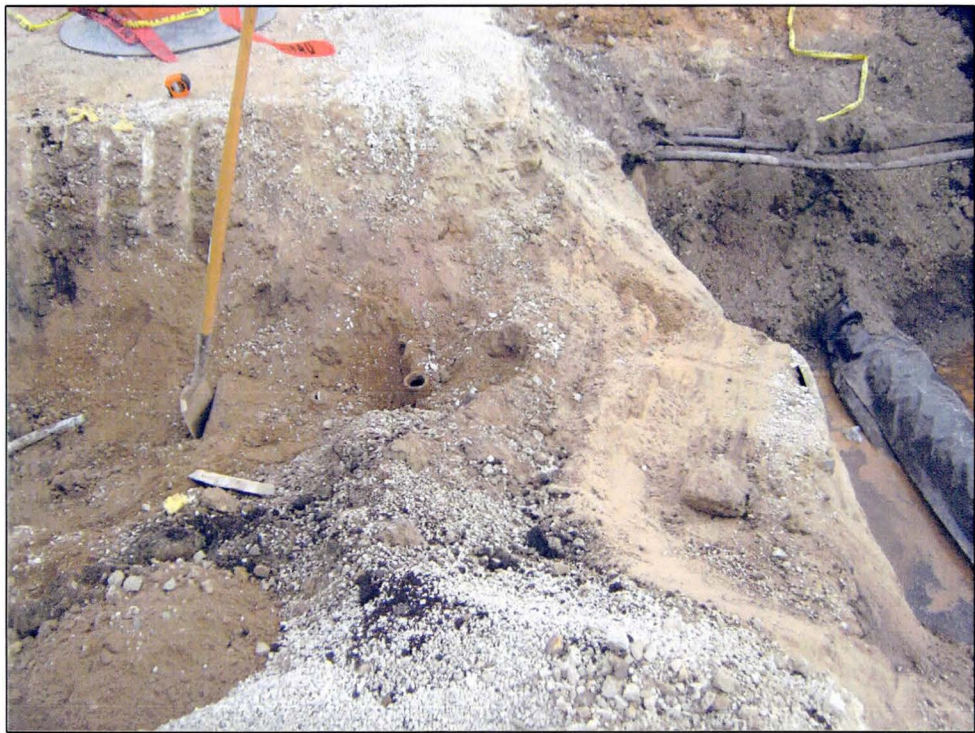
Photo 4 – Location of UST in Relation to Water Line and High Voltage Underground Electric Lines
