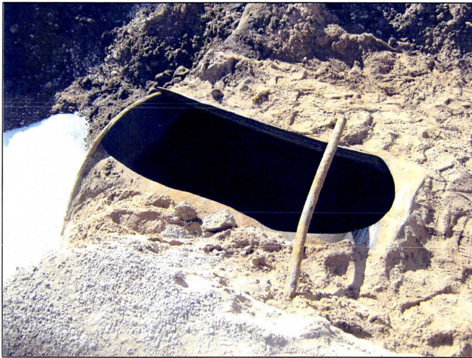
Photo 7 – Hole in UST for Cleaning.
