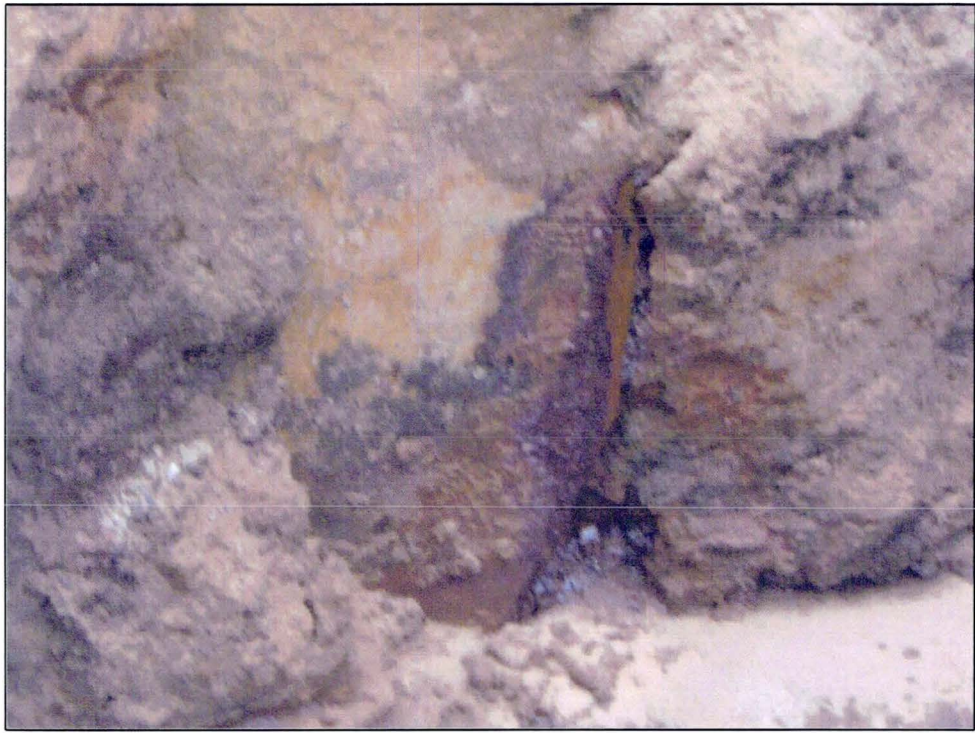
Photo 3 – Soil Staining Adjacent to UST.
