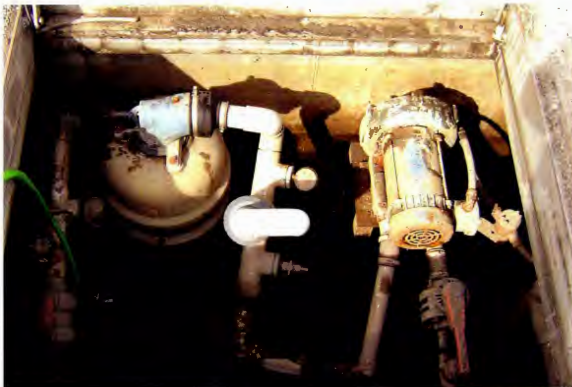
PHOTOGRAPH 4: VELR System #1 pre-decommissioning.
