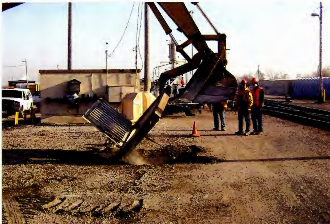
PHOTOGRAPH 5: VELR System #2 lid being removed.
