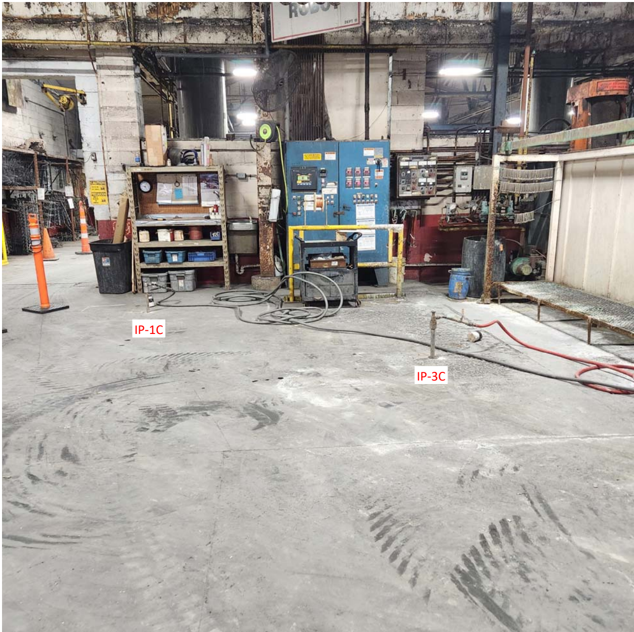
Photo #2. View of typical injection points connected to individual hoses delivering the solution. Injection points IP-1C and IP-3C are visible, facing north.
