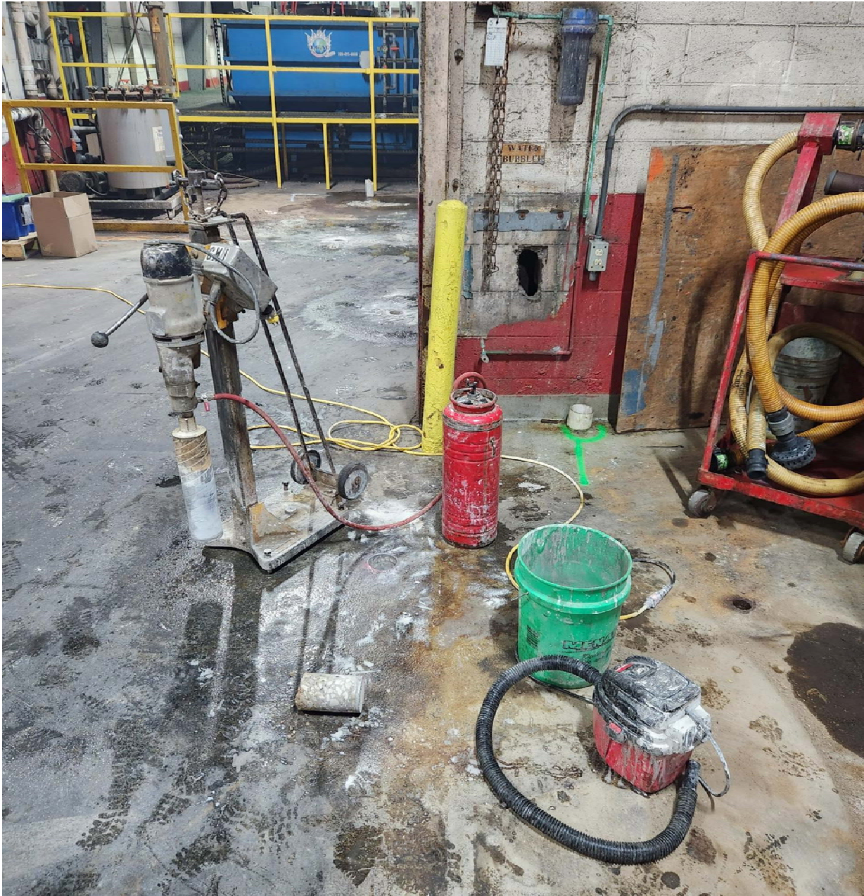
Photo #1. Concrete coring was completed at each injection point inside the facility in preparation for advancement of the direct-push tooling.
