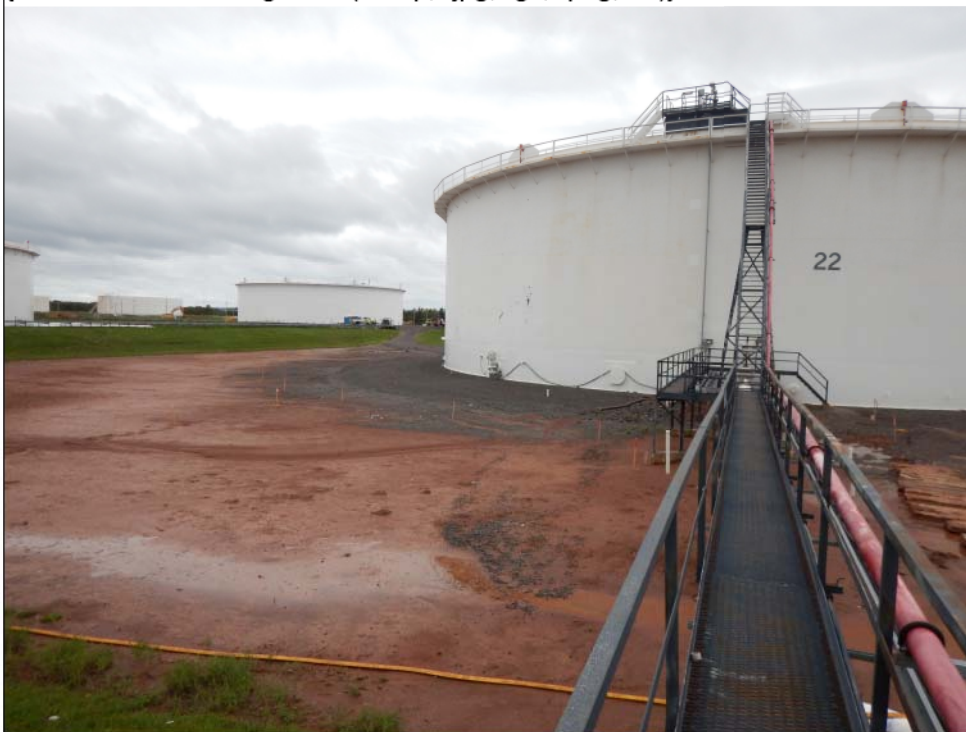
Title: Enbridge Energy Tank 22 looking NW
