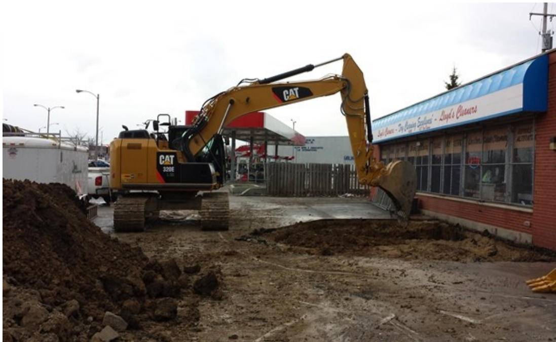
Above: Excavating top 3-4 feet of non-hazardous soil. Rain off and on during remedial excavating.
