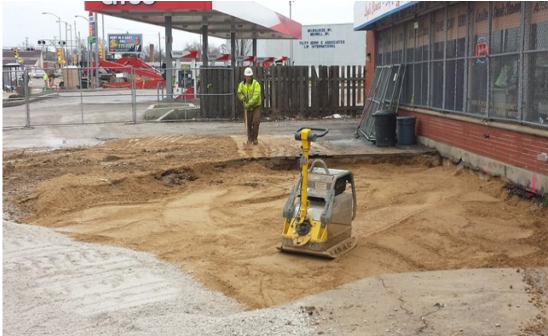
Above: Final compacting of fill and placement of crushed dolomite base material (traffic bond) for restorative paving.
