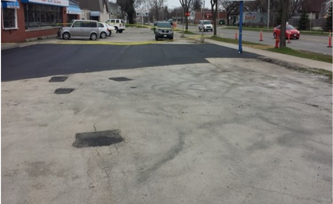
Above: Restoration of asphalt paving and replacement of concrete sidewalk squares complete.
