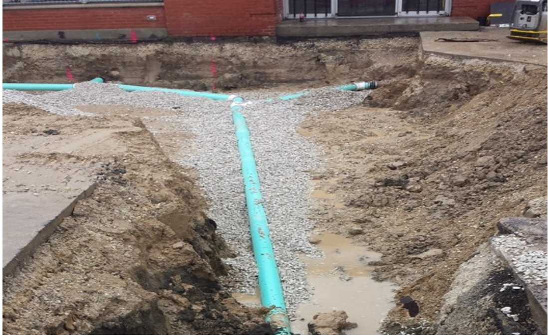
Above: Permanent storm sewer lateral laterals with roof drain laterals connected on right and left-hand sides of the picture.
