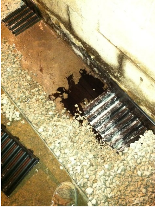
Above and Below: Black oily substance identified as 10-weight oil observed seeping out of the basement block wall through weep holes (weep hole visible in mid-right of photo above, and upper right of photo below). Note staining in joints of concrete block.
