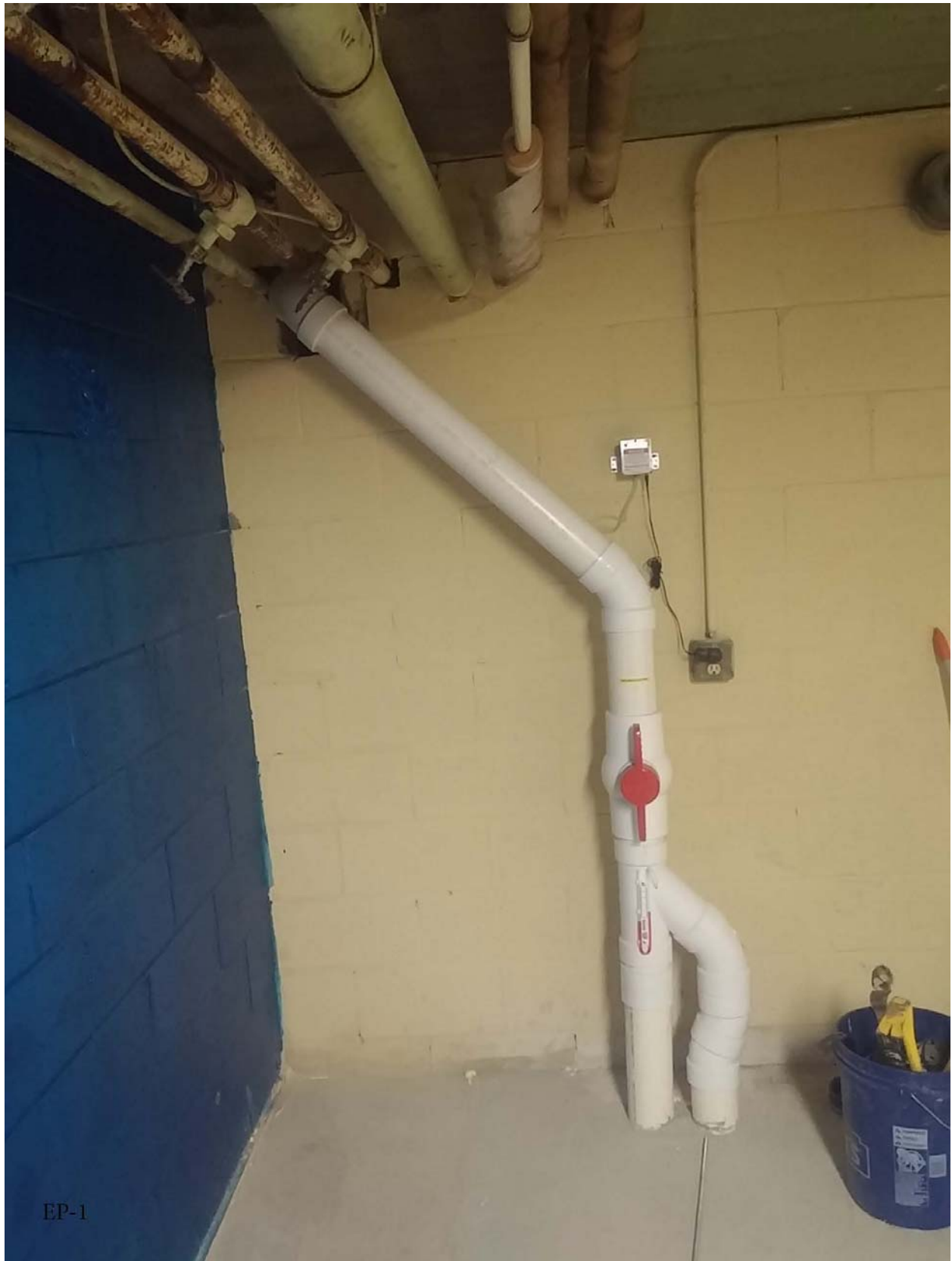
SSDS extraction points at north end of main storage room.
