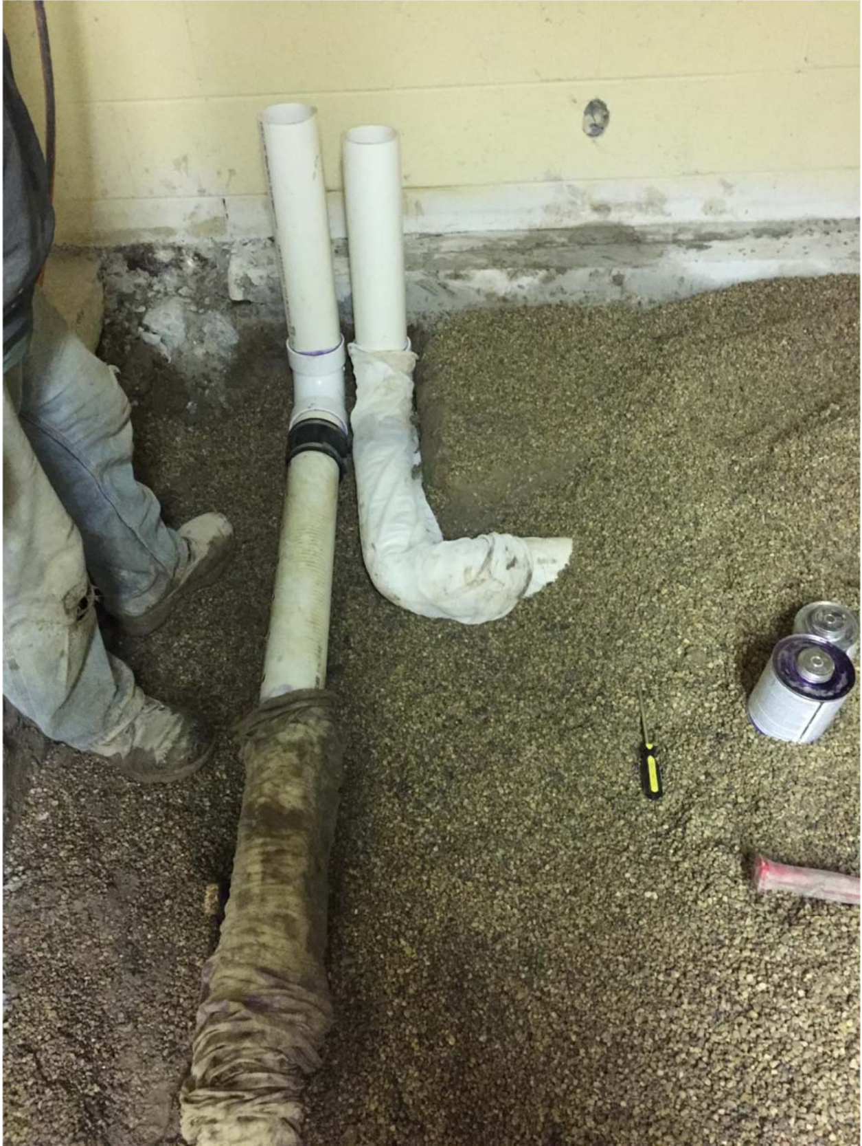
Vent pipe risers. Facing north.
