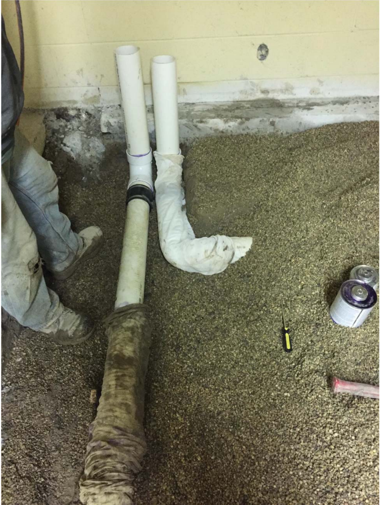
Vent pipe risers. Facing north.
