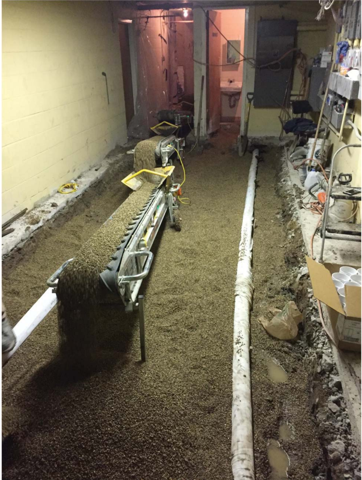
Horizontal vent pipes and pea gravel backfill in main storage room. Facing south.
