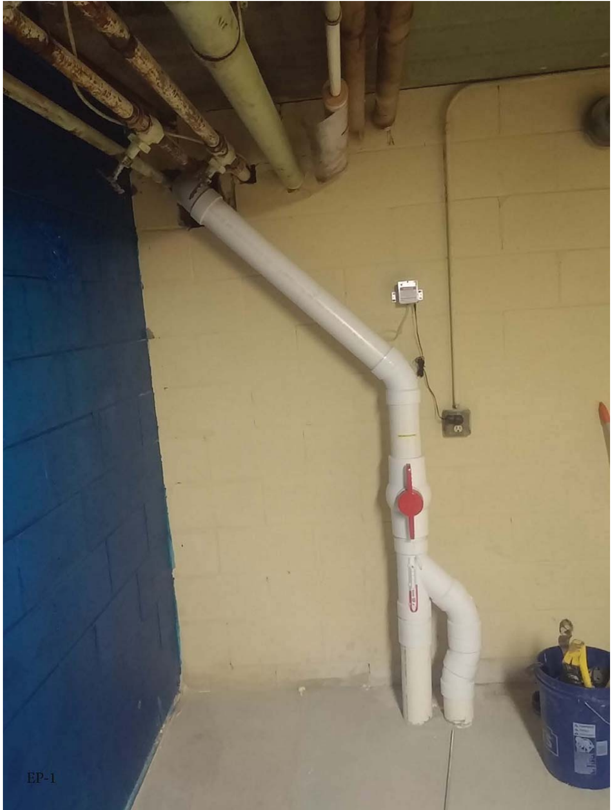
SSS extraction points at north end of main storage room.
