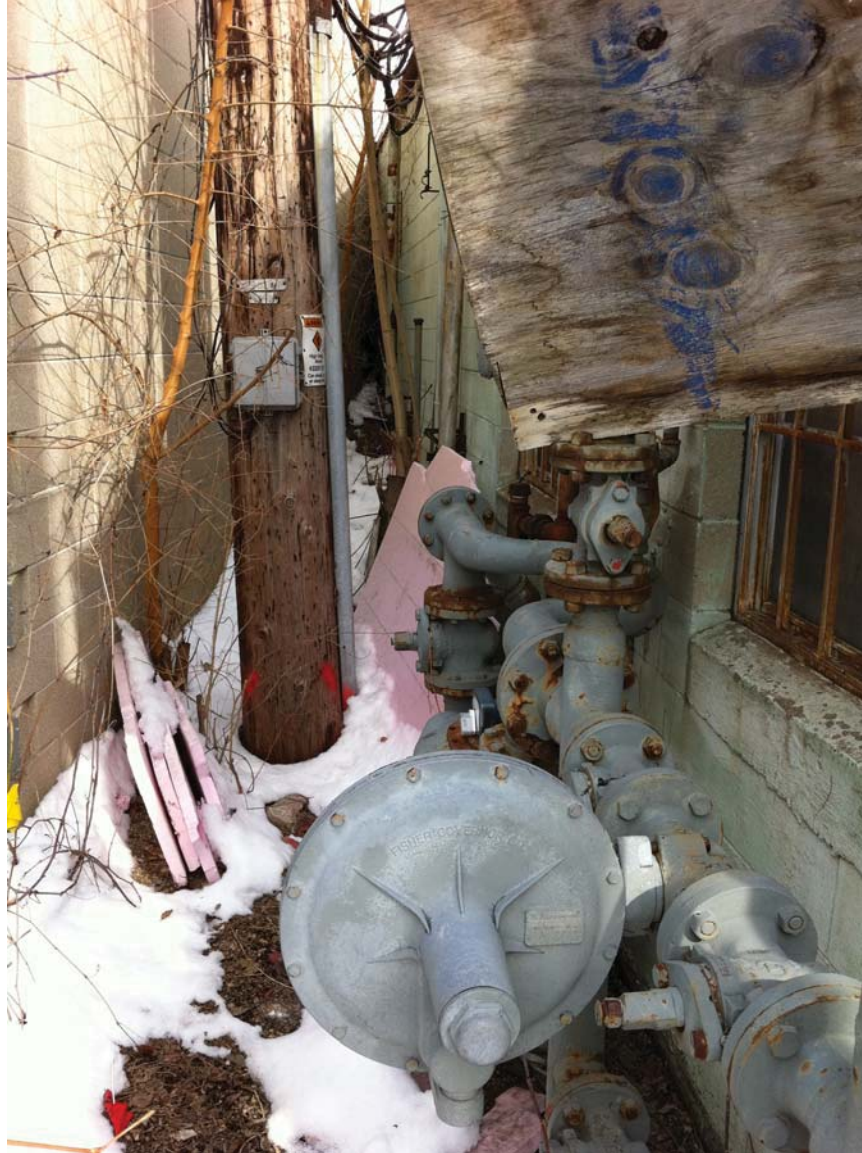
Natural gas and electrical utility infrastructure creating a structural impediment for remediation between the west wall of the Site building and the beighboring Benz Oil building.
