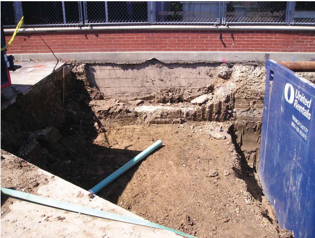
The western boundary of the exterior excavation was the footing for the slab on grade portion of the building. The building was a structural impediment for remediation under the floor slab.
