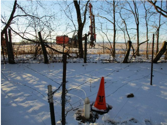
Photo #1 Photo looking south at MW-6 with drill rig set-up at MW-9 location, 100 feet to south in field.
