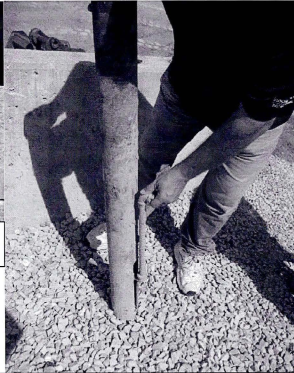
4) 4-inch pipe "sleeved" over 1-inch line valve.
