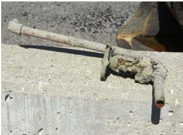
3) 1-inch pipe & valve that was connected to 10-inch line underground
