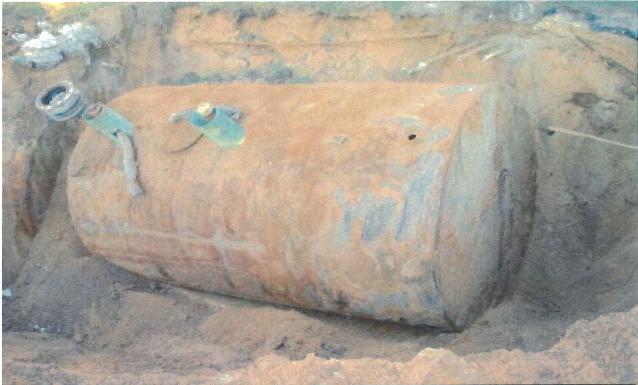
Photograph the 6,000 gallon unleaded gasoline underground storage tank.
