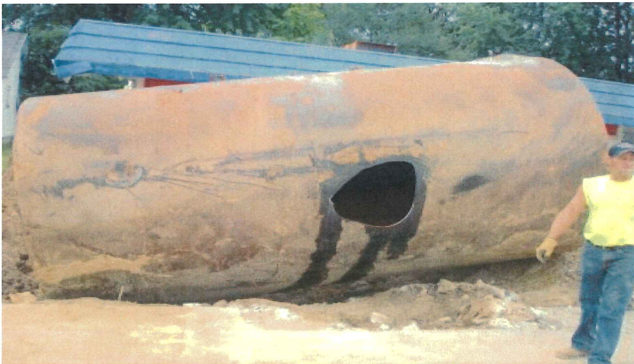
Photograph of the 8,000-gallon unleaded gasoline underground storage tank.
