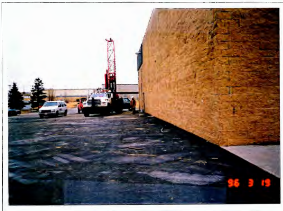
Installation of soil boring. Please observe that asphaltic concrete covers former UST area.
