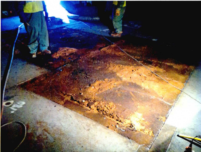
Photo 7: Tank 23 bottom cut-out. Petroleum contaminated fill sediment with surficial discoloration (darker coloration) shown. January 31, 2013
