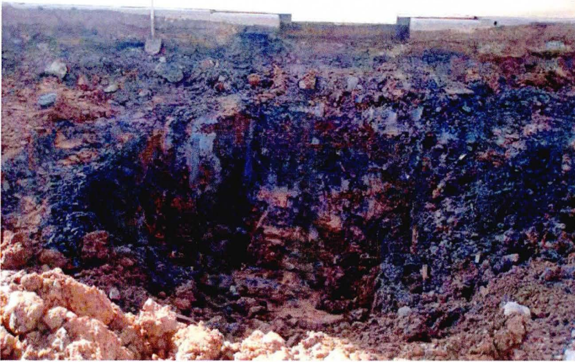
Photo 3: Contaminated soil near northern D-door. April 9, 2012.
