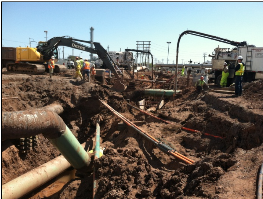
Photo 6: The cement conduit and impacted soil were removed during hydrotest excavation activities.
