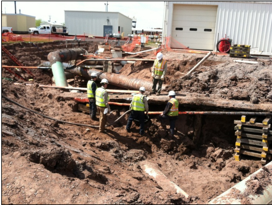
Photo 5: Cement conduit with crude oil impacted soil beneath it.
