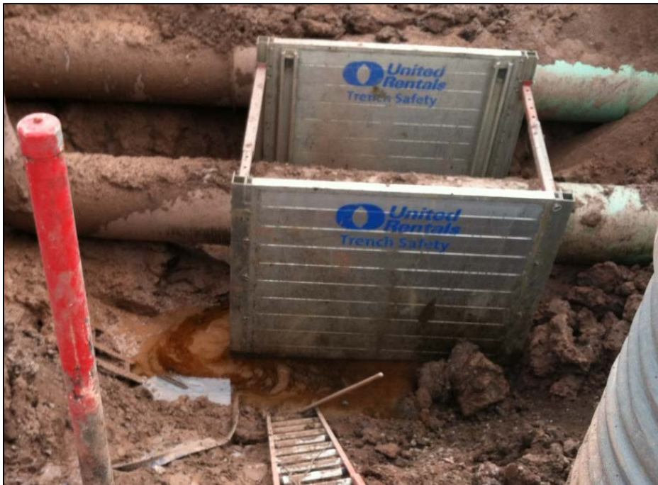
Photo 4: Water in the hydrotest excavation with crude oil on the surface. Crude oil impacted water was observed in the east end of the excavation near the 6-BV-1 valve. Water was containerized in frac tanks and treated at the City of Superior Environmental Services Division of Public Works (ESDPW) facility.
