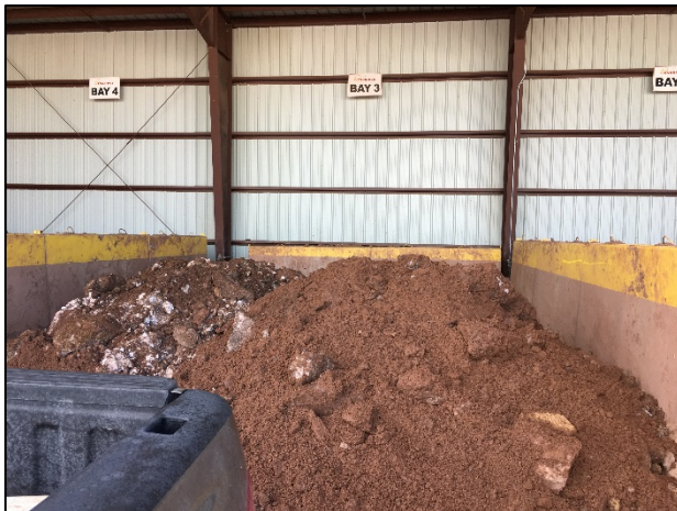
Photo 11: Excavated soil from the Line 6 pipeline trap tie-in stockpiled in the Superior Terminal SMA. Photo taken on February 13, 2017.
