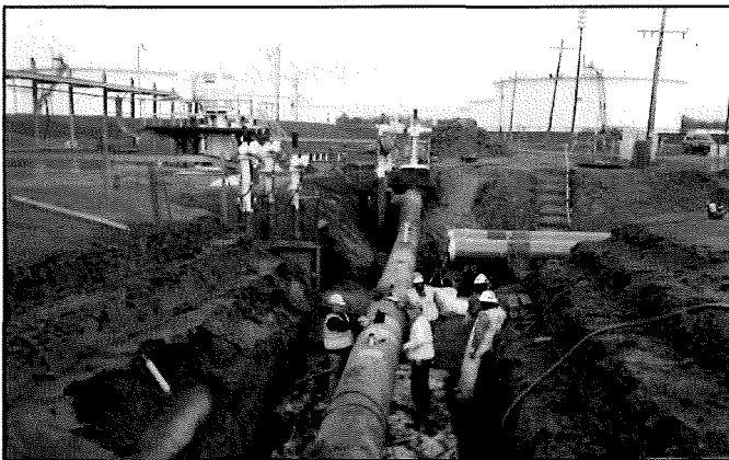
Photo 1: Line 14 (center of photo) maintenance excavation, facing northeast. The valves with historical crude oil impacts soil are shown on the left side of Line 14. Photo taken on October 28, 2013.
