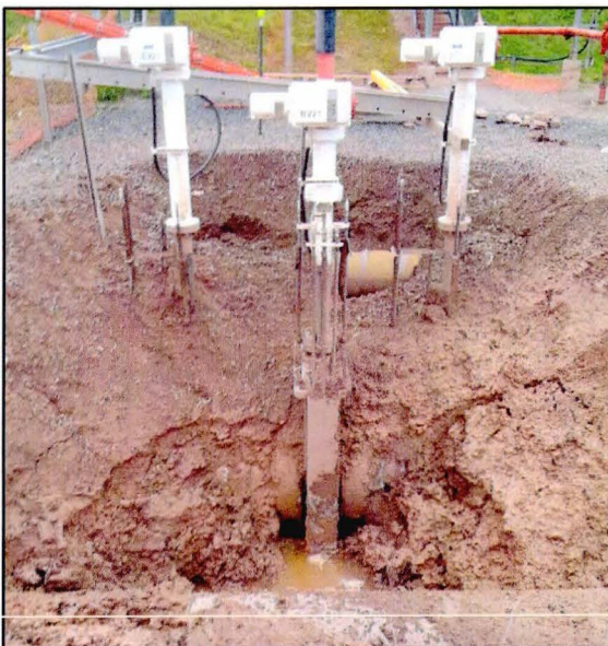
Photo 2: Water with sheen encountered in excavation during hydrovac excavation activities. These valves were the location of the 2011 crude oil release (BRRTS #0216558992) that was closed by the WDNR in 2012. Photo taken on October 23, 2013.
