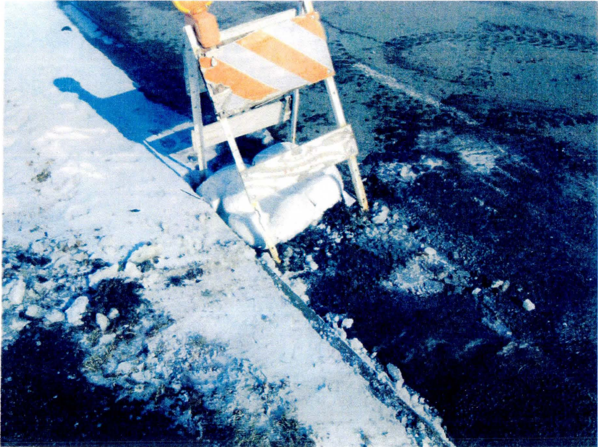
Storm Sewer with Absorbent Boom Placed
