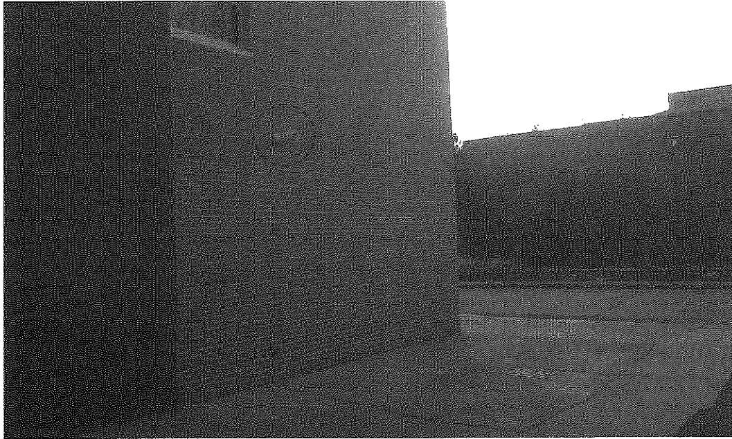
Photo 15: 4" PVC subslab vent system exhaust point at west wall in the south half of the building (view to southeast; December 2, 2014).
