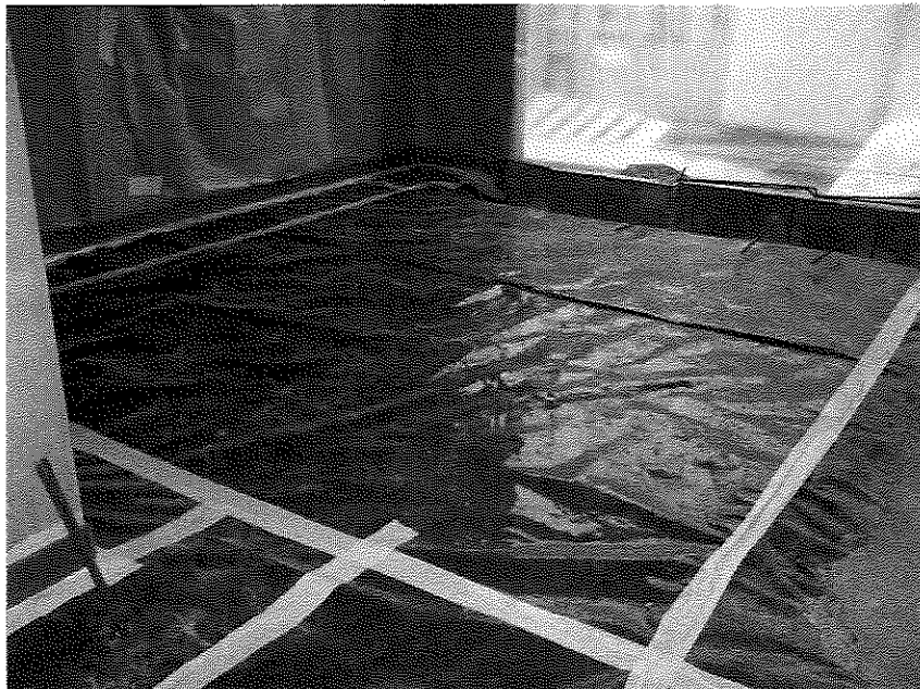
Photo 2: 15-mil vapor barrier in process of being installed in northeast portion in north half of building with taped seams and perimeter (view to east-northeast; March 12, 2014).
