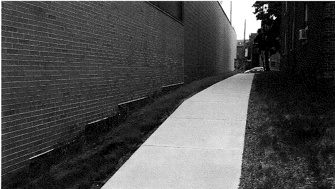
Photo 20: Exterior of north side of building with concrete sidewalk and grass on neighboring property to the right (view to west; June 12, 2015).
