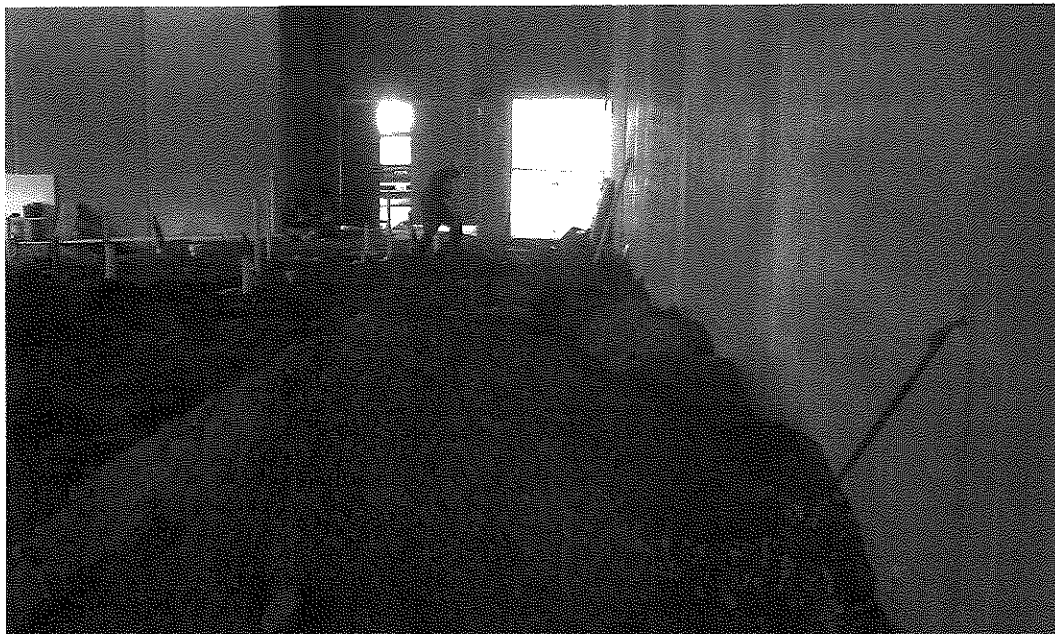
Photo 6: Typical trench dug into base course layer in the south half of building (background) and sandy gravel stockpile to be used as backfill around subslab vent pipe (foreground) (view to west; June 19, 2014).
