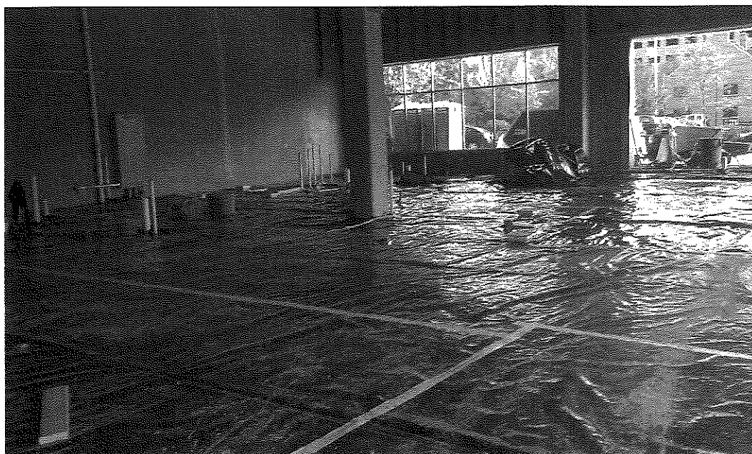
Photo 11: 15-mil vapor barrier in process of being installed at east end in south half of building with taped seams and perimeter (view to northeast; October 3, 2014).
