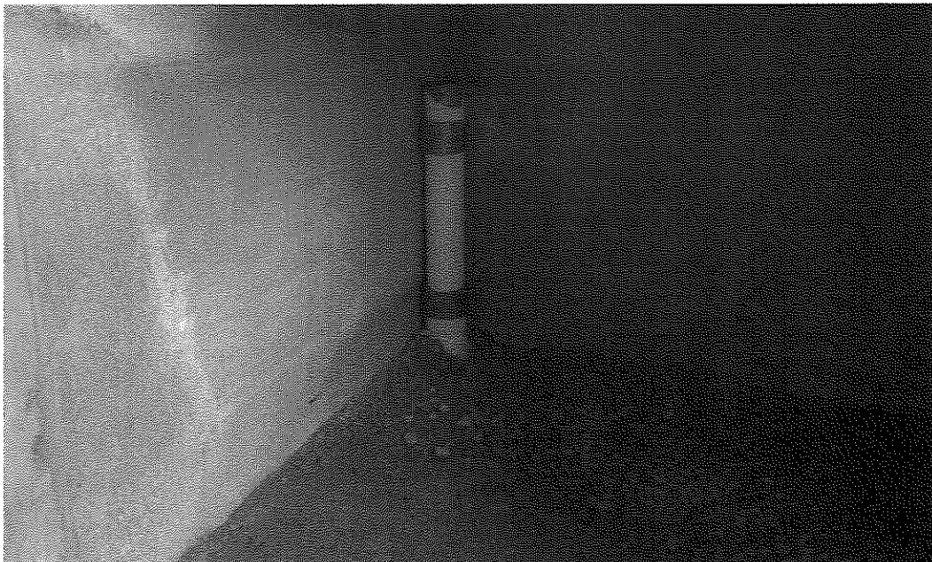
Photo 8: 4" PVC pipe stub for subslab vent system exhaust point at west wall in the south half of the building (view to northwest; June 30, 2014).
