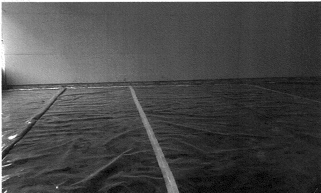
Photo 10: 15-mil vapor barrier in process of being installed in central portion of south half of building with taped seams (view to west; October 2, 2014).
