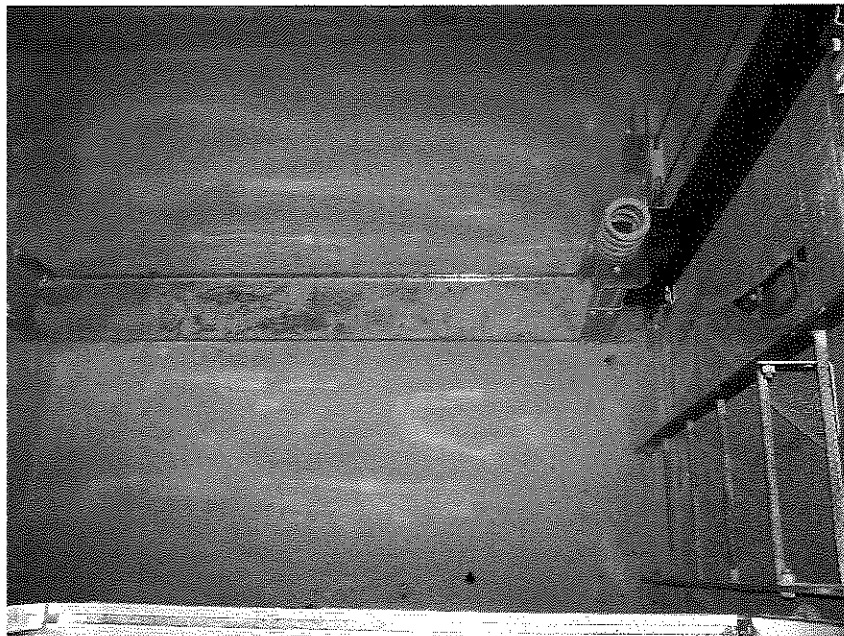
Photo 24: Vapor proofing material (Perm-A-Barrier Liquid) installed on base (and walls) of west elevator pit in the northeast portion of the building (facing north; February 6, 2015).
