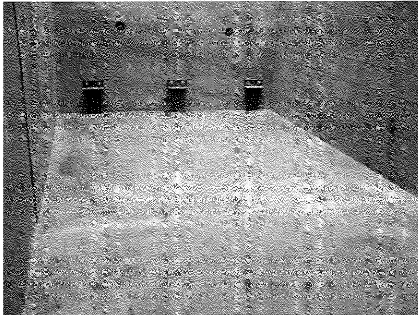
Photo 4: Concrete floor slab installed over vapor barrier in north stairwell in north half of building (view to west; March 7, 2014).
