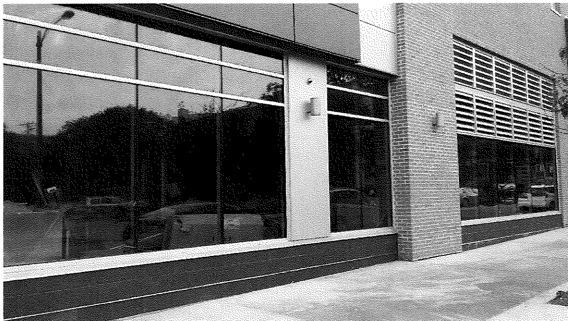
Photo 18: 4" PVC subslab vent system exhaust point at east wall in the south half of the building after vent cover installed (view to northeast; June 12, 2015).
