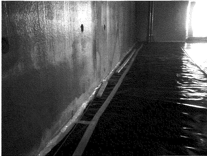
Photo 1: 15-mil vapor barrier in process of being installed in north-central portion in north half of building with taped seams and perimeter (view to east; March 7, 2014).
