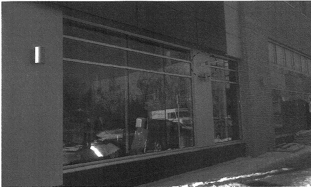
Photo 17: 4" PVC subslab vent system exhaust point at east wall in the south half of the building (view to northwest; January 15, 2015).
