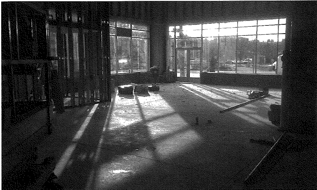
Photo 13: Concrete floor slab installed over vapor barrier in south half of building for retail areas on first floor (view to southeast; December 2, 2014).
