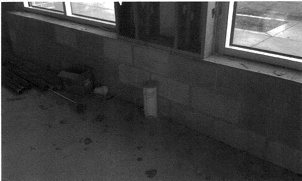
Photo 14: 4" PVC pipe stub for subslab vent system exhaust point at east wall in the south half of the building (view to northeast; December 2, 2014).
