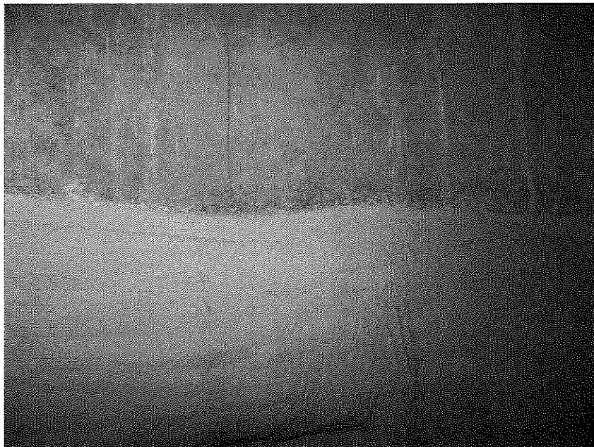
Photo 26: Close-up view of vapor proofing material (Perm-A-Barrier Liquid) as installed in elevator pits in the northeast portion of the building (February 6, 2015).
