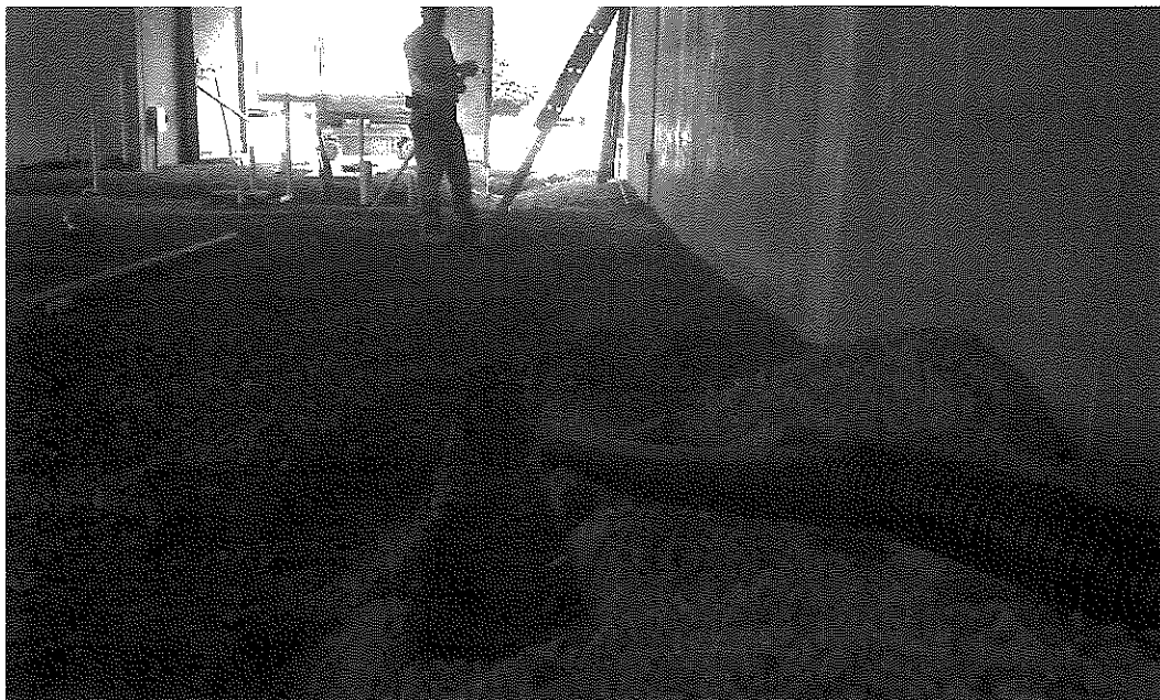
Photo 7: Typical 4-inch diameter perforated subslab vent pipe in process of being installed in south half of building for passive subslab vent system (view to west; June 30, 2014).
