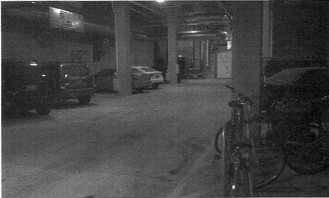
Photo 5: Concrete floor slab installed over vapor barrier in north half of building for parking garage (view to west-southwest; January 15, 2015).
