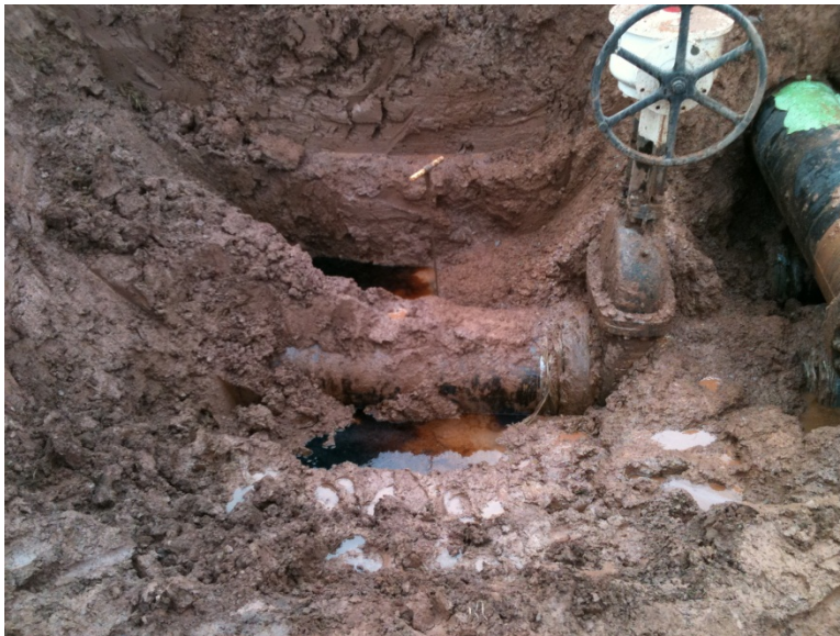
Photo 1: Early valve repair excavation. Addition excavation work was required to locate the leak and complete the repairs. (4/6/2011)
