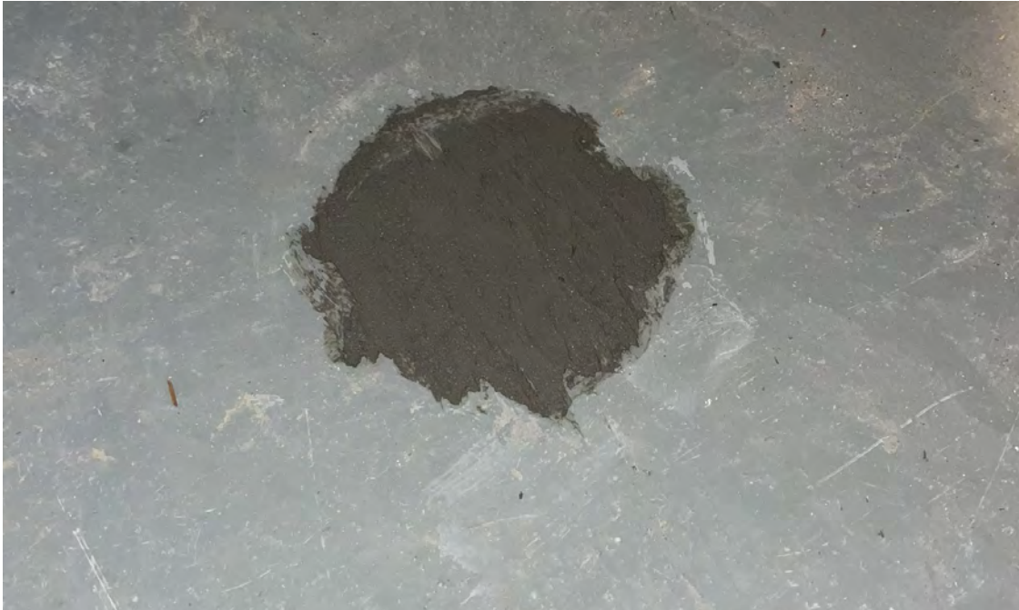
Photo 15: Filled and sealed location of SSV-01 in 122912th Avenue building following passive sampler retrieval. 3/29/2023.
