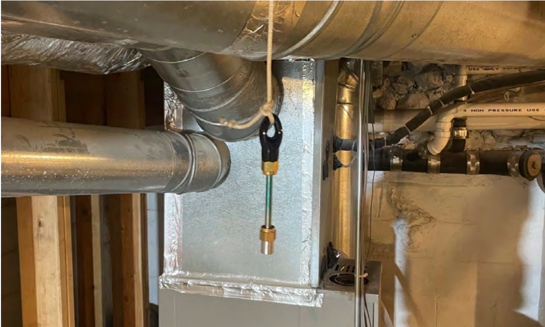
Photo 9: Indoor air sampler installed in basement of 1229 12th Avenue building. 3/22/2023.
