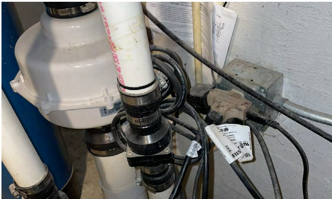
Photo 16: Reactivated vapor mitigation system in 1229 12th Avenue building. 3/29/2023.
