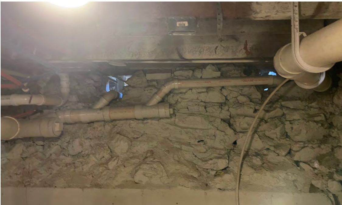
Photo 2: View of west basement wall in 1229 12th Avenue building. View to west. 3/8/2023.
