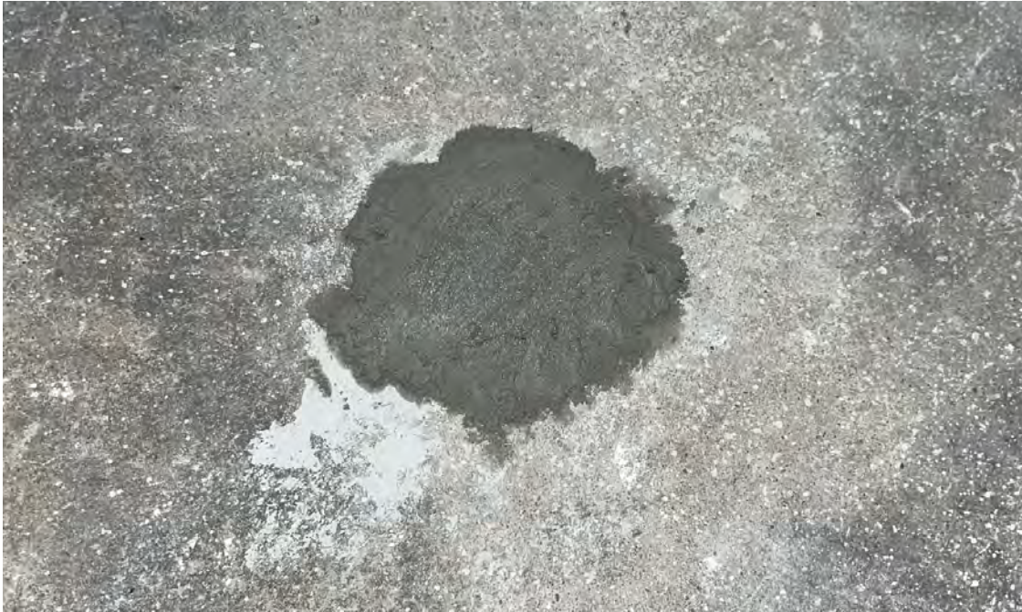
Photo 13: Filled and sealed location of SSV-02 in 1233 12th Avenue building following passive sampler retrieval. 3/29/2023.
