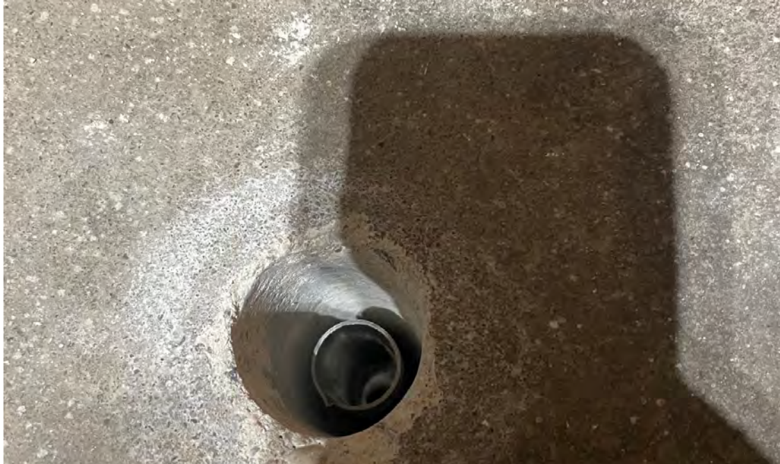
Photo 6: Sub-slab sample point SSV-03 in the 1233 12th Avenue building following installation of the aluminum tube. 3/22/2023..
