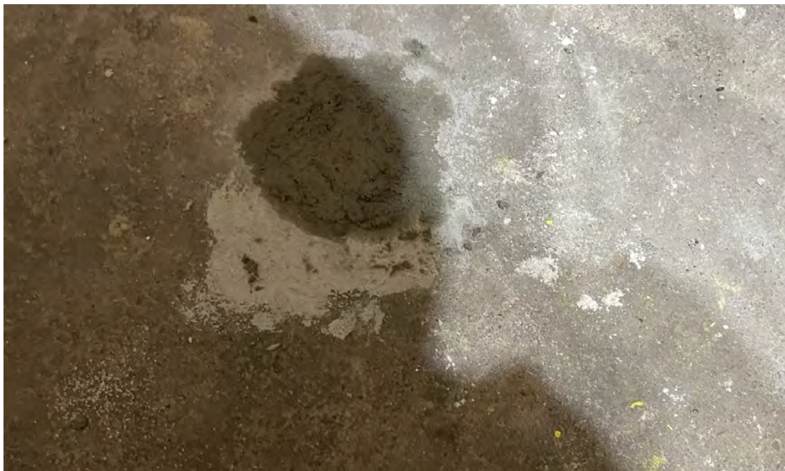
Photo 14: Filled and sealed location of SSV-03 in 1233 12th Avenue building following passive sampler retrieval. 3/29/2023.
