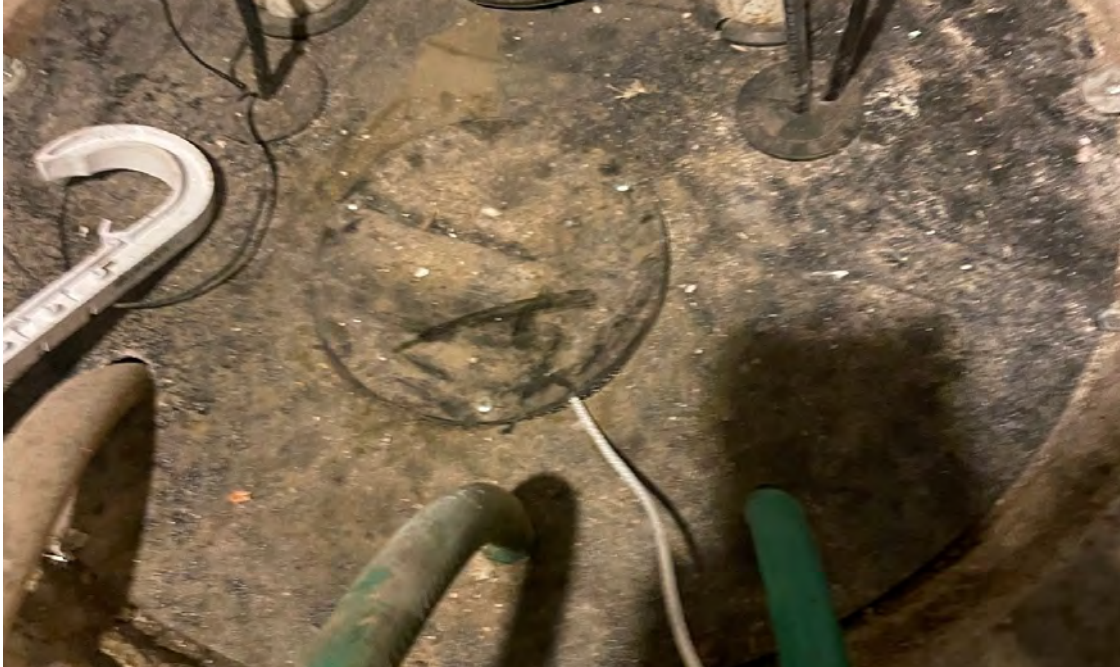
Photo 6: Passive sampler installed in headspace of basement sump in the 1229 12th Avenue building. 3/22/2023.
