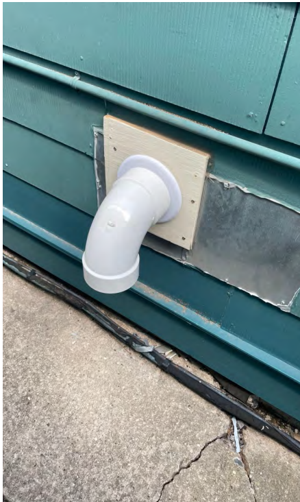
Photo 6: View of mitigation system discharge on north exterior of 1229 12th Avenue building. 3/8/2023.
