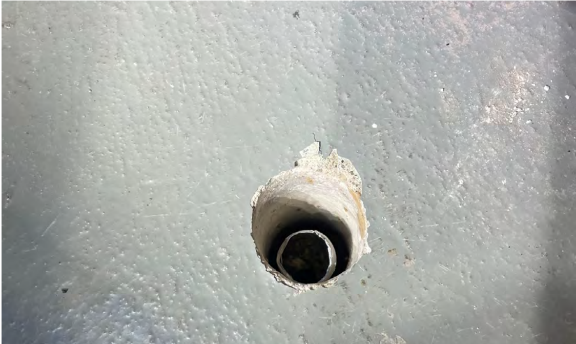
Photo 1: Sub-slab sample point SSV-01 in the basement of the 1229 12th Avenue building following installation of the aluminum tube. 3/22/2023
