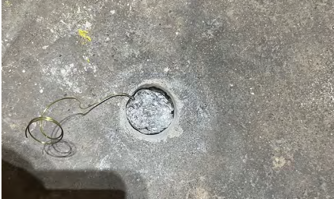
Photo 4: Sub-slab sample point SSV-02 in the 1233 12th Avenue building following installation of the passive sampler and aluminum foil plug. 3/22/2023
