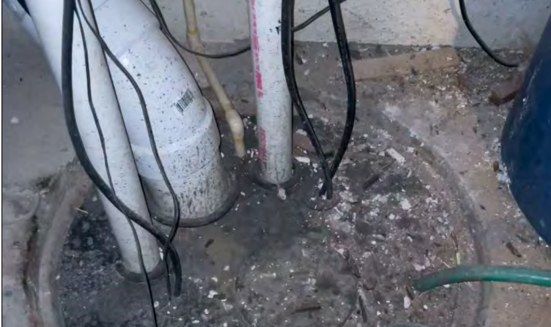
Photo 4: View of sump in basement of 1229 12th Avenue building. 3/8/2023.
