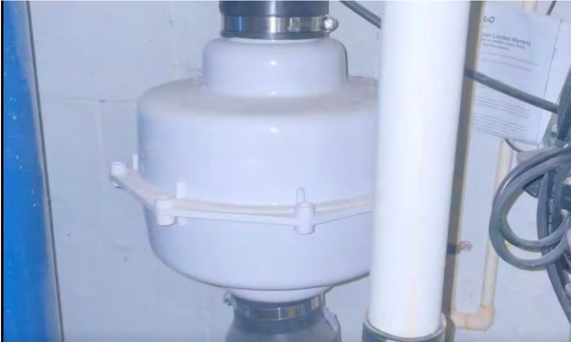
Photo 5: View of mitigation system fan connected to sump in 1229 12th Avenue building. 3/8/2023.
