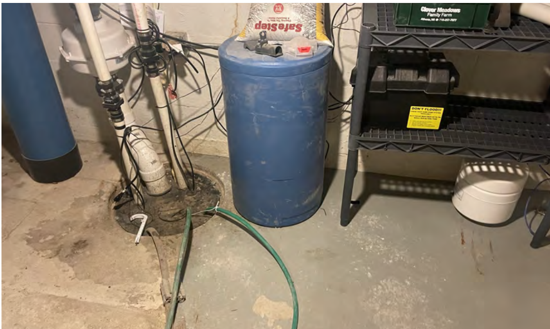
Photo 12: View of sealed sump in basement of 1229 12th Avenue building prior to retrieval of sampler from sump headspace. View to north. 3/29/2023.
