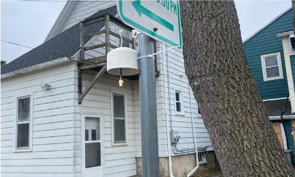
Photo 11: Ambient air sampler installed to the west of the 1229 12th Avenue building. View to northeast. 3/22/2023
