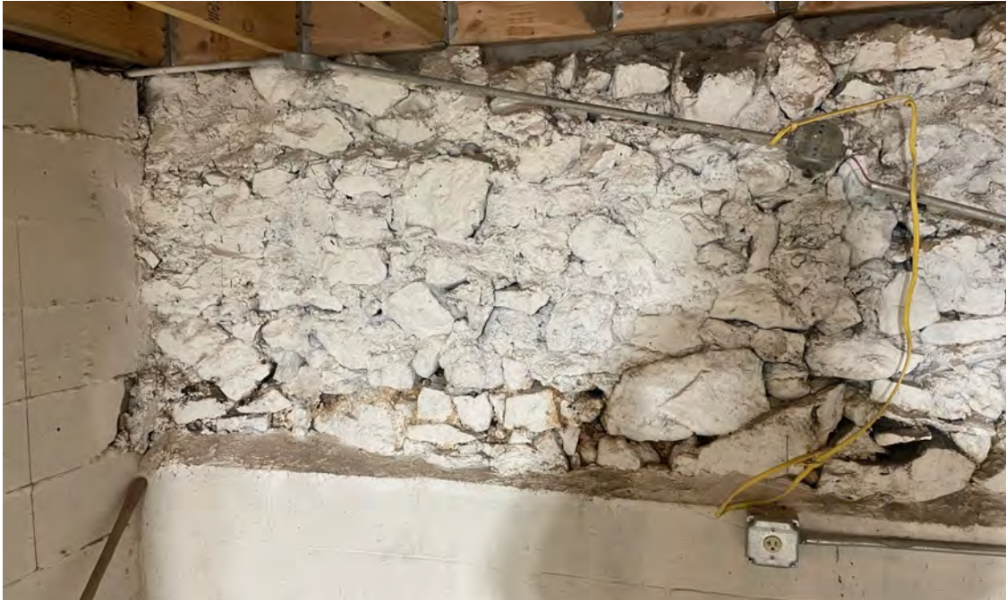
Photo 1: View of eastern portion of north basement wall in 1229 12th Avenue building, View to north. 3/8/2023.
