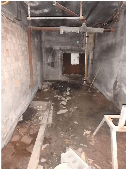
Interior view of earthen floor room looking south with contaminated soil and debris.
