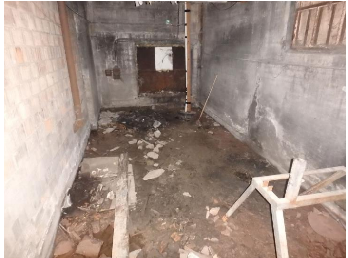
Another view of basement room subject to corrective action.
