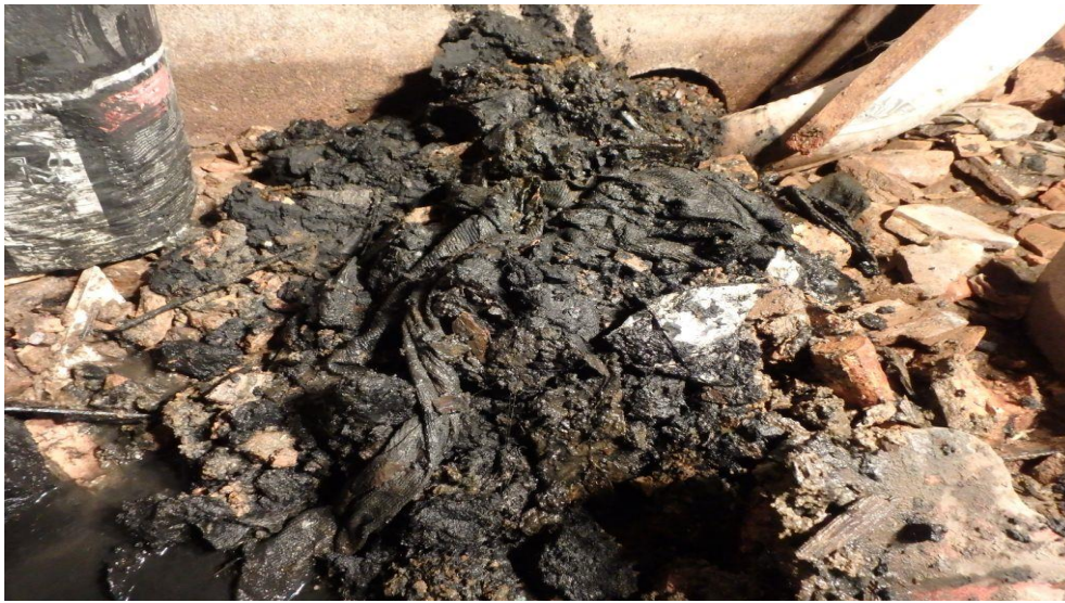
Closeup of contaminated media encountered during initial removal activities.
