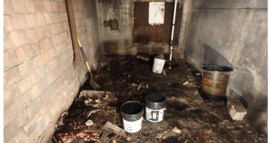
View of basement room prior to cleanup in January 2017.
