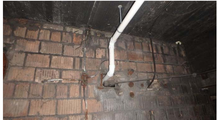
Sealed holes in wall
