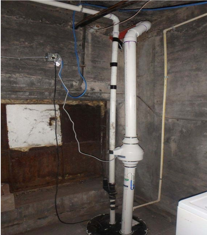
View of Radon System
