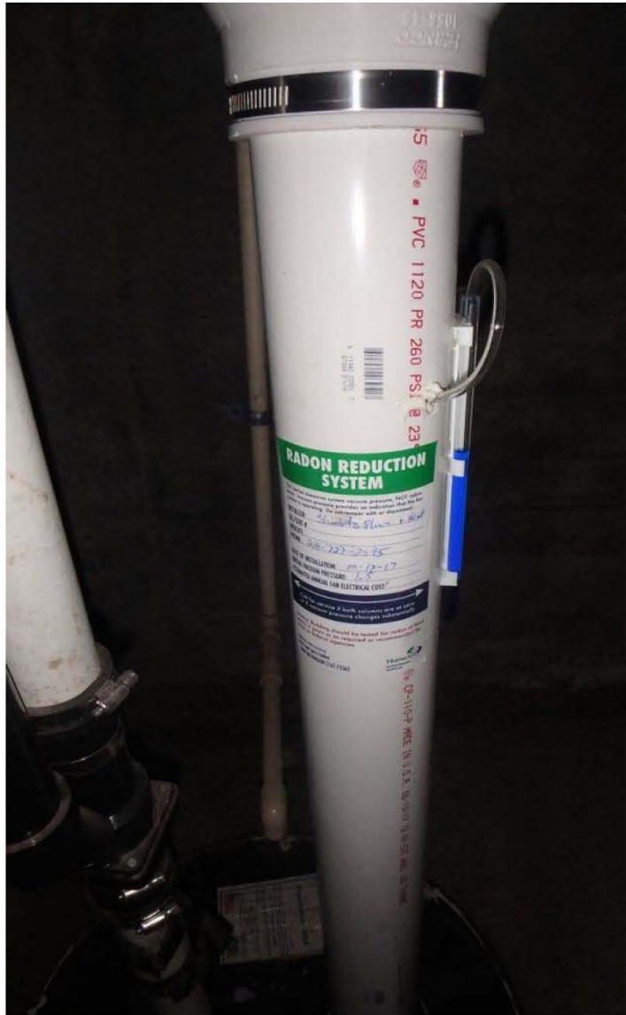
Close up of piping
