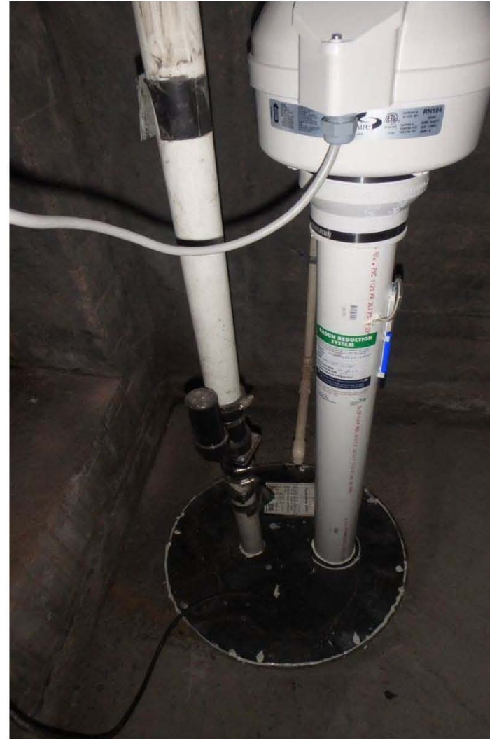
Close up of Radon System and sump
