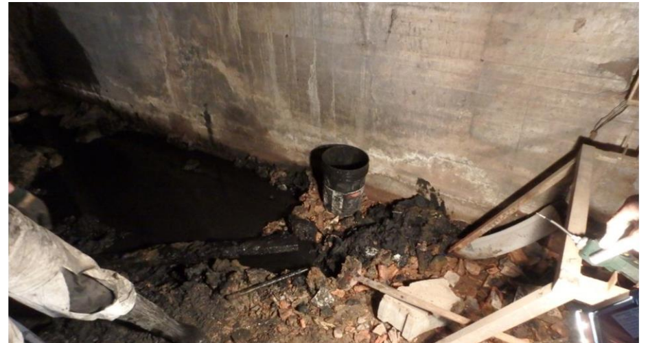
View of area where sump was installed prior to cleanup in January 2017.
