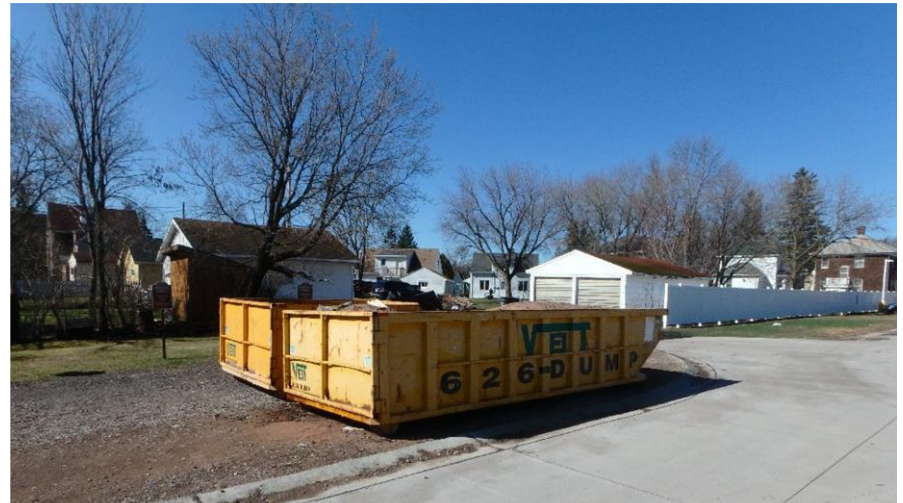
View of roll off containers on site prior to hauling off site for disposal.
