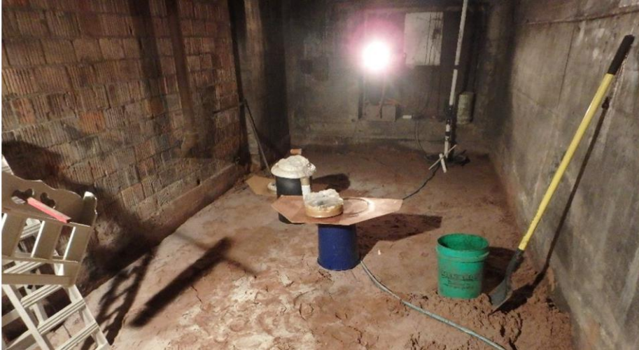
View of basement room area after cleanup activities took place in March 2017.
