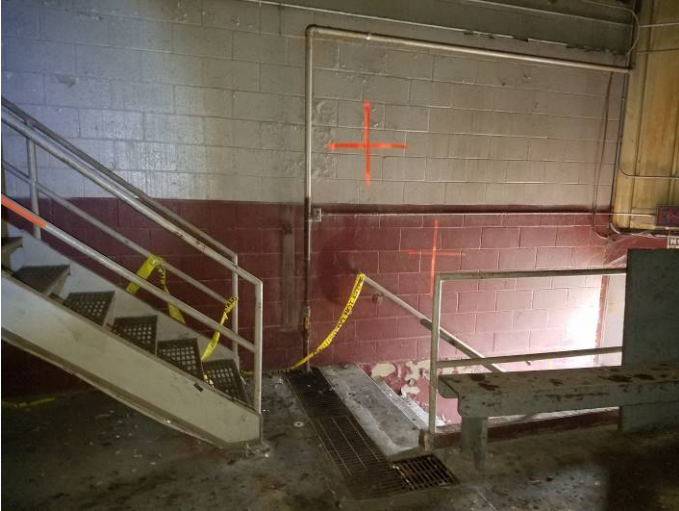
Photo 21) Typical Wall with Lead-Based Paint
