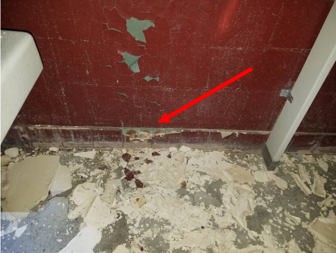
Photo 19) Brown Ceramic Baseboard Adhesive - Bldg 9 Bathroom
