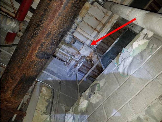
Photo 7) Typical Pipe Fitting Insulation
