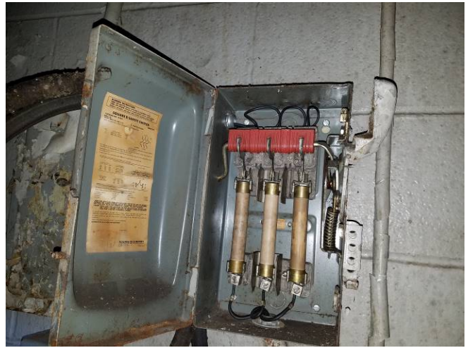
Photo 11) Typical Electrical Panel
