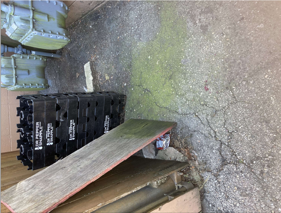
Title: Asphalt cap with some cracks, north side of the building near the back exit.
