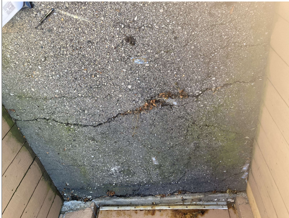
Title: Crack in the asphalt cap on the north side of the building near the fencing around the dumpster.
