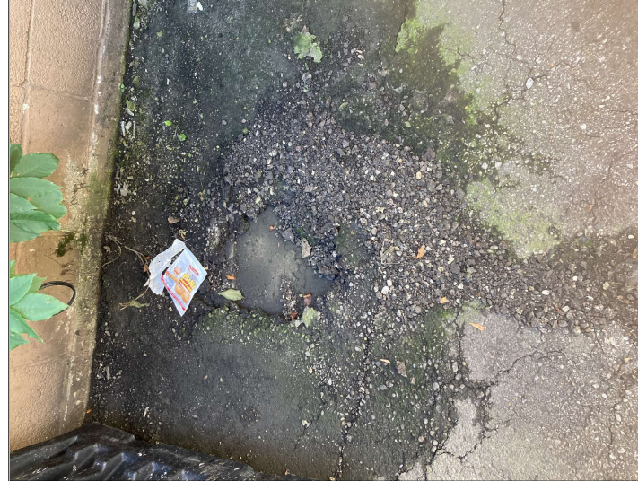
Title: Asphalt degraded cap ~1' x 1' inside of fence near dumpster.
