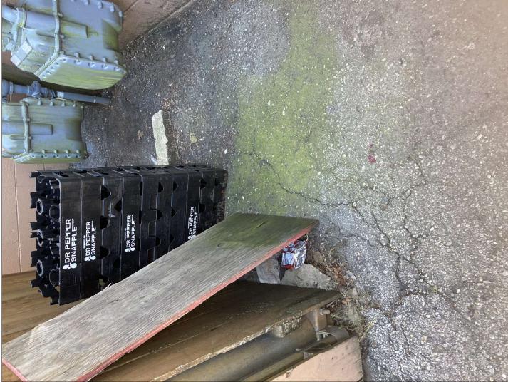
Title: Cracks in the asphalt cap, north side of building near the dumpsters.
