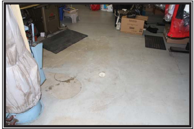
Photo 2 Typical view of slab on grade floor of the buildings on Site.
