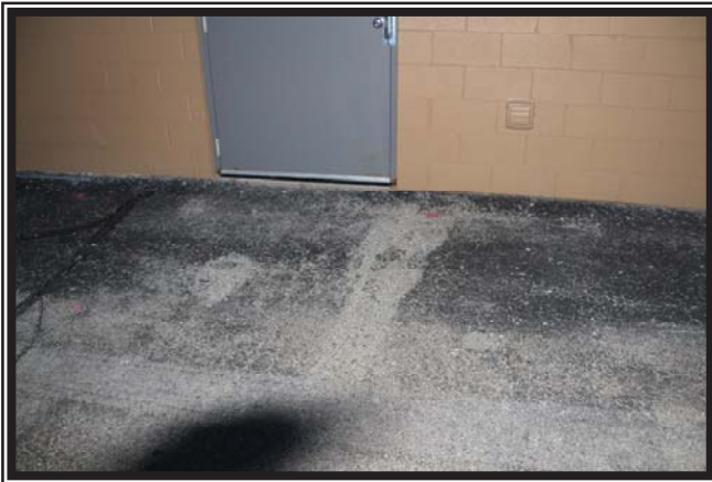
Photo 3 View of asphalt cover over drive directly outside of Rainbow Cleaners unit.
