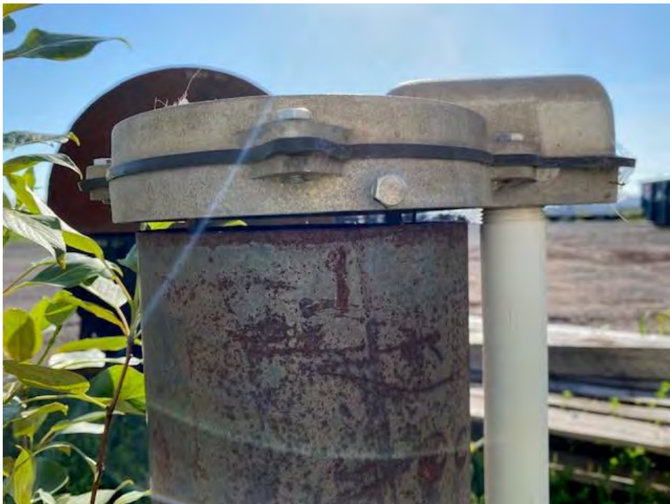
Photo 2: Gap between PW-2 well casing and cover.
