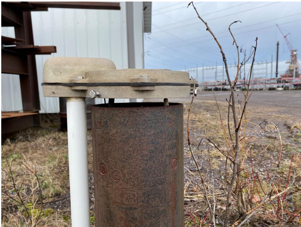
Photo 2: Gap between PW-2 well casing and cover.
