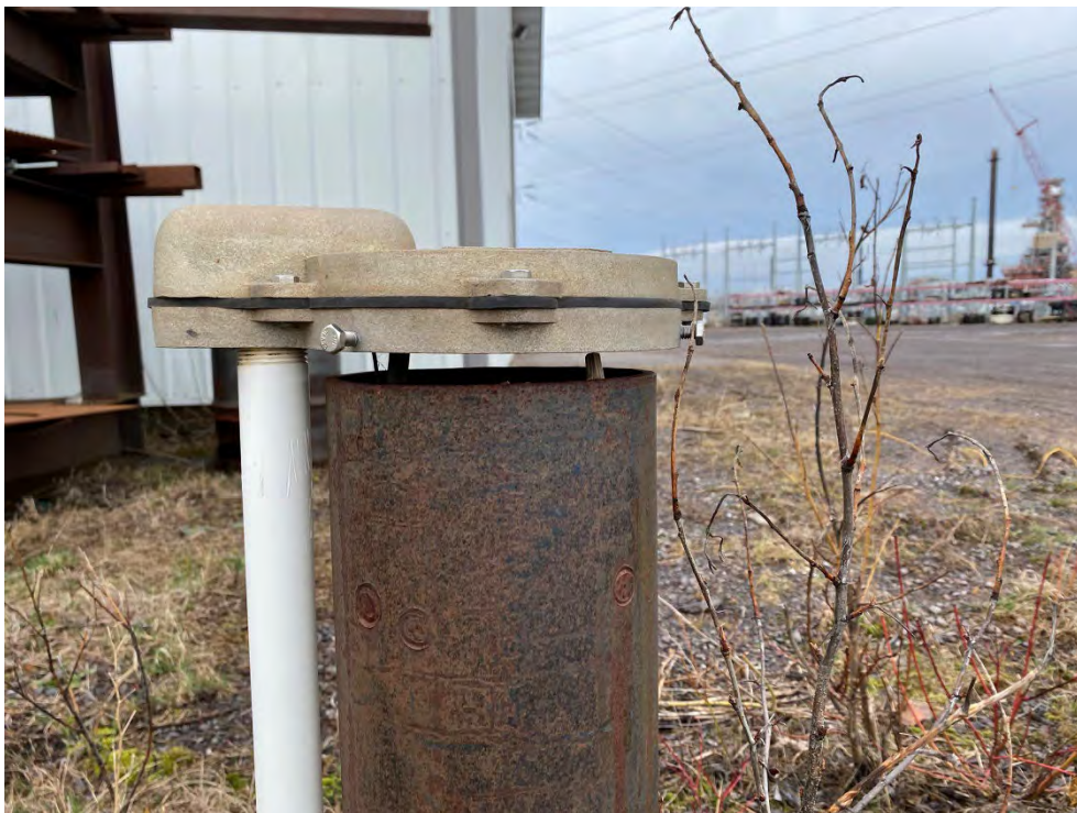
Photo 2: Gap between PW-2 well casing and cover. (May 12, 2022)
