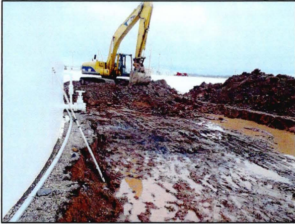
Photo 5: The road construction excavation on the southeast corner of Tank 8 near the water draw-off valve.
