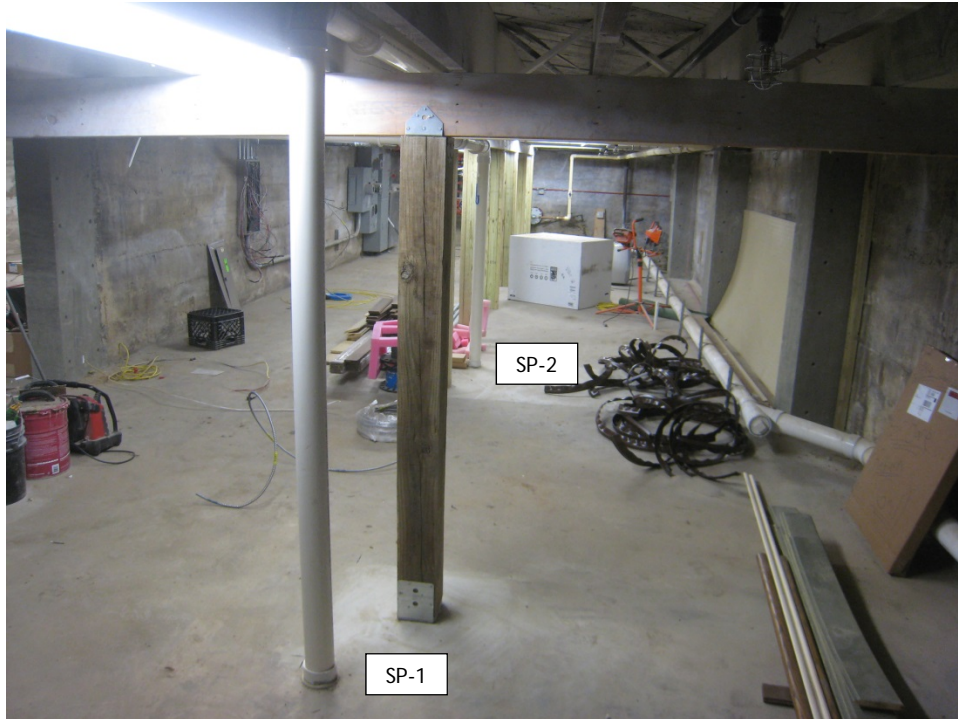
Vapor Mitigation System and Soil Cap in basement at the 2536 address. Two floor penetrations are installed at this address (West U-Tube location). Looking southeast, photo taken 2/5/15.
