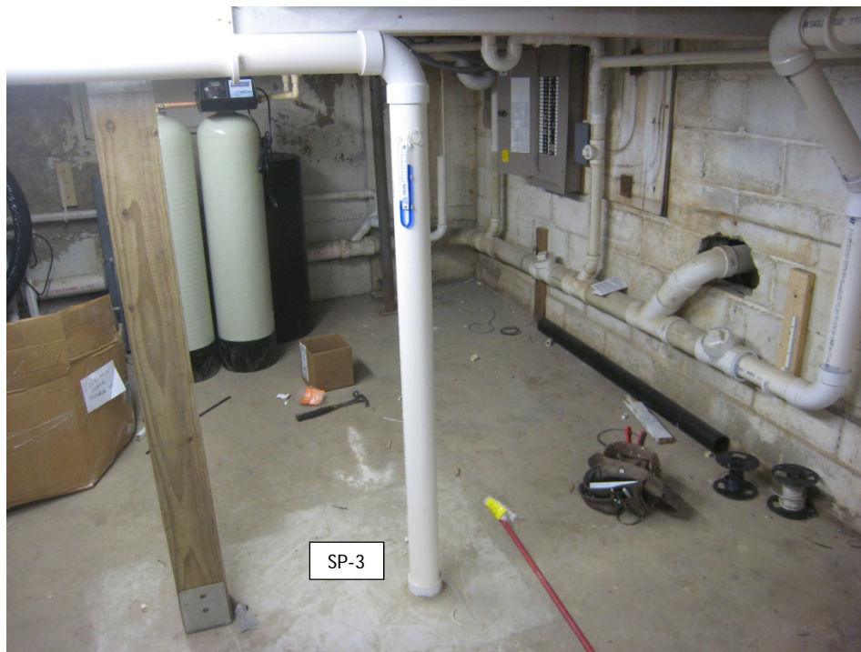
Vapor Mitigation System and Soil Cap in basement at the 2534 address. One floor penetration is installed at this address (Central U-Tube location). Looking north, photo taken 2/5/15. Note: The U-Tube should look as pictured in photo, with one side of the fluid higher than the other if fan is functioning properly. If fluid levels are equal, fan is not operating.
