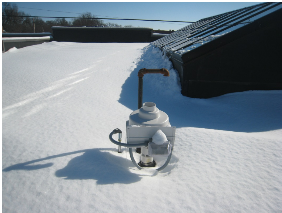
One of two high vacuum fans (RadonAway GP501) located on building roof (2536 Monroe St.). This fan exhausts subslab vapors from the 2534 and 2536 address. The other fan exhausts vapors from the 2532 address. Looking southeast, photo taken 2/5/15.
