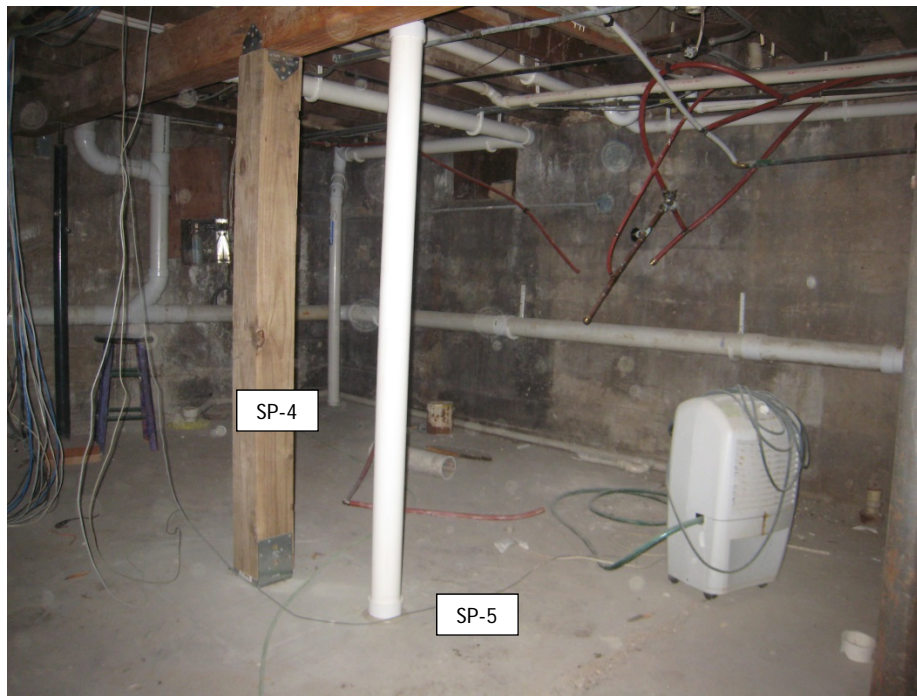
Vapor Mitigation System and Soil Cap in basement at the 2532 address. Two floor penetrations are installed at this address (East U-Tube location). Looking west, photo taken 2/5/15.
