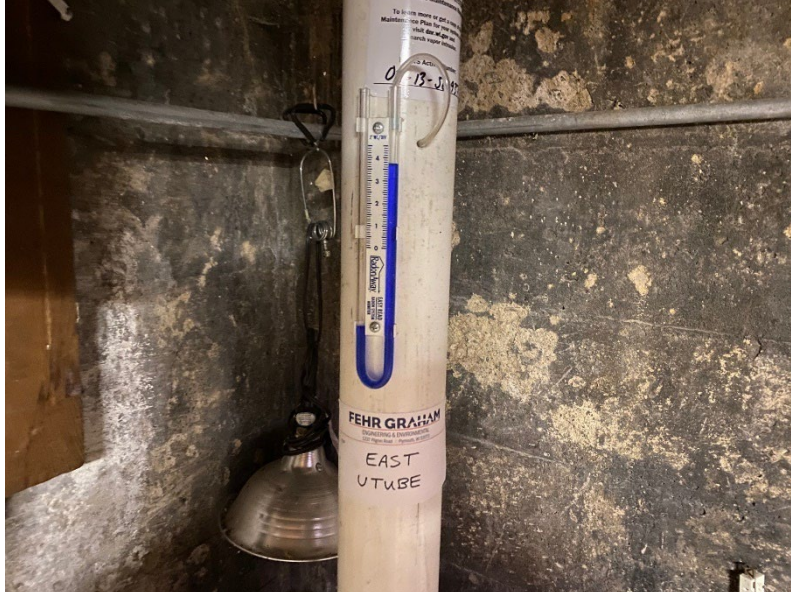
5. Properly working East U-Tube Manometer, facing northwest.
