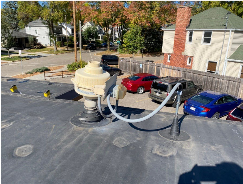
10. Second high vacuum fan (RadonAway GP501), facing northwest.
