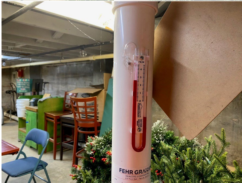
2. Newly installed West U-Tube Manometer, facing south.
