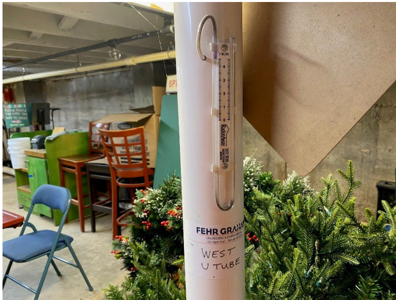
1. Damaged West U-Tube Manometer, facing south.
