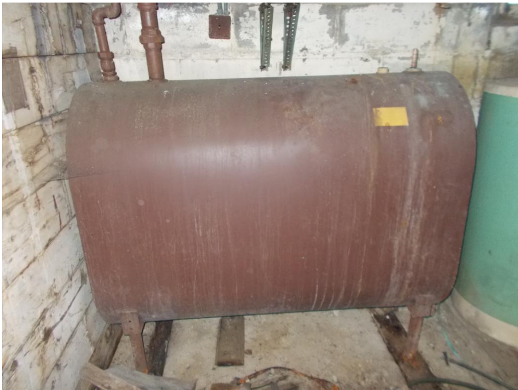
7) View of the AST located in the basements
