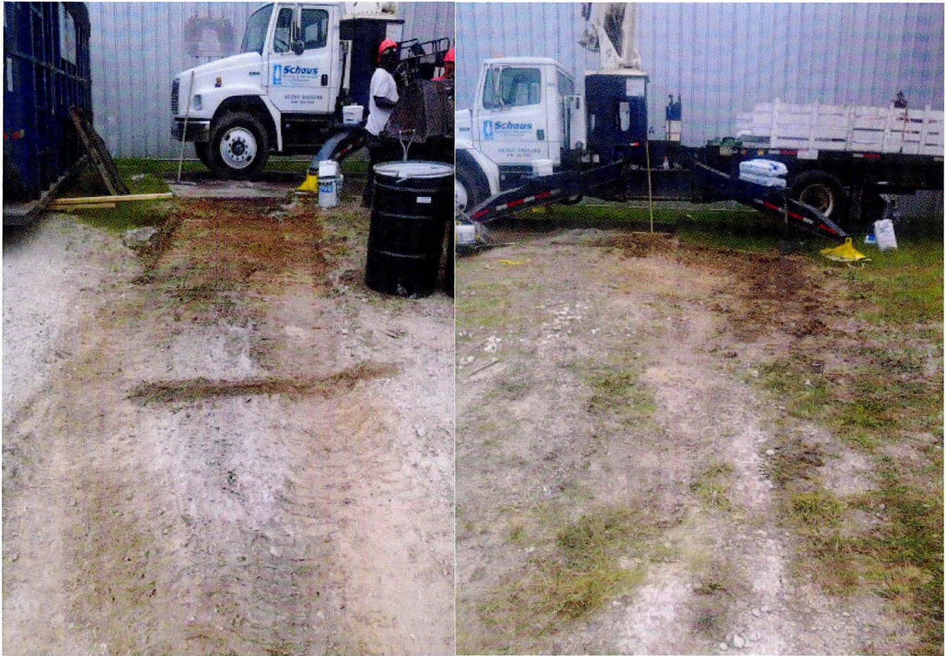
Top 3 pictures show spill containment on concrete slab. Pictures 4-8 show clean-up efforts with oil absorbents. Pictures 9 & 10 show gravel removal efforts in-progress.
